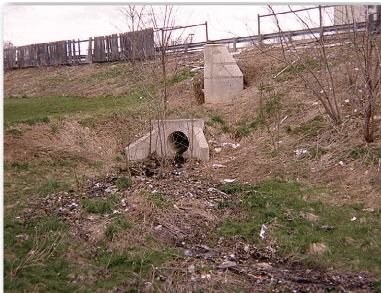
Storm water in a city is usually collected in storm sewers and transported to a stream in large pipes. This photo shows water exiting a pipe into a stream.
