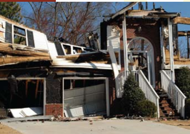
Explosion and fire damage caused by the volatile chemicals used in a meth lab.
