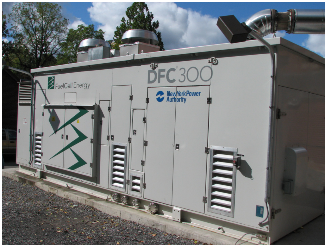
Figure 1-1. FuelCell Energy DFC 300A Molten Carbonate Fuel Cell at SUNY-ESF
