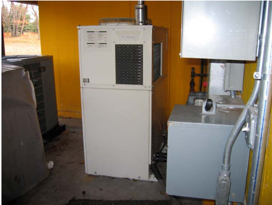
Figure 1-1. Current Installation of Aisin Seiki G60 Cogeneration Unit at Hooligans
