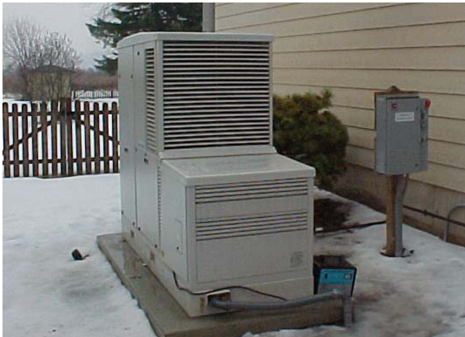
Figure 1-2. The SU1 System at the Lewiston Residence
