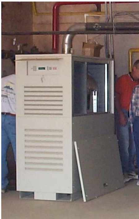
Capstone 30 kW Microturbine
