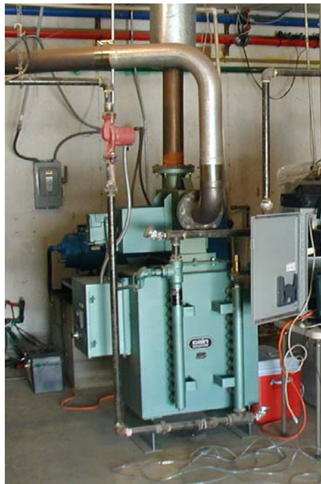
Cain Industries Heat Recovery System
