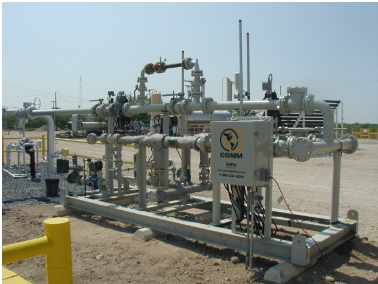
Figure 1-4. The Installed COMM EVRU System
