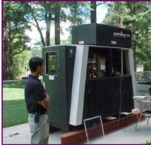
Figure 1-2. The Turbogenerator at the College Park BCHP Test Facility
