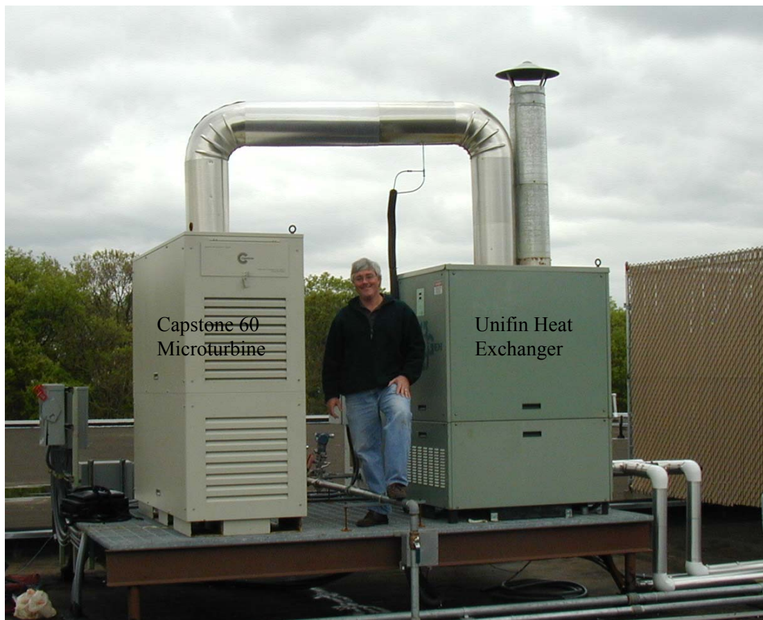
Figure 1-1. The Waldbaum's Capstone 60 Microturbine System
