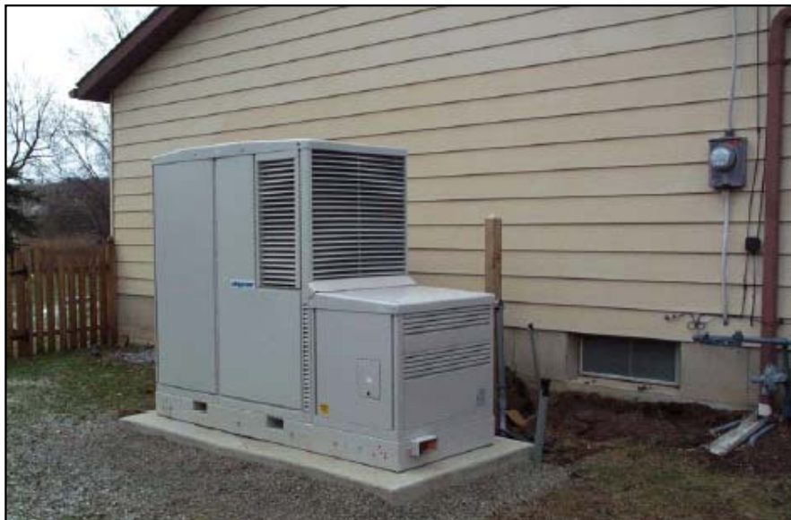
Figure 1-2. Plug Power SU1 System Installed at the Host Site in Lewiston, NY
