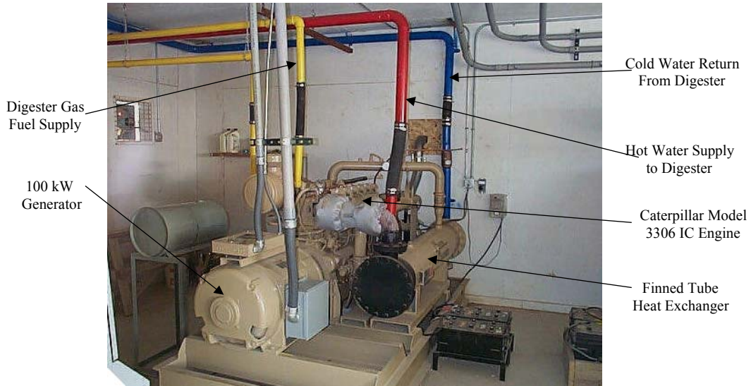
Figure 1-4. Colorado Pork IC Engine CHP System
