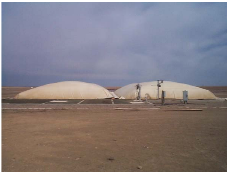
Figure 1-6. Colorado Pork Anaerobic Digester
