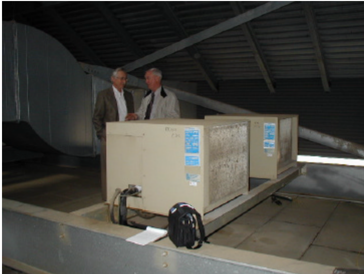
1 1/2 hp single compressor, refrigerant charge of 15.11 lbs R-502
