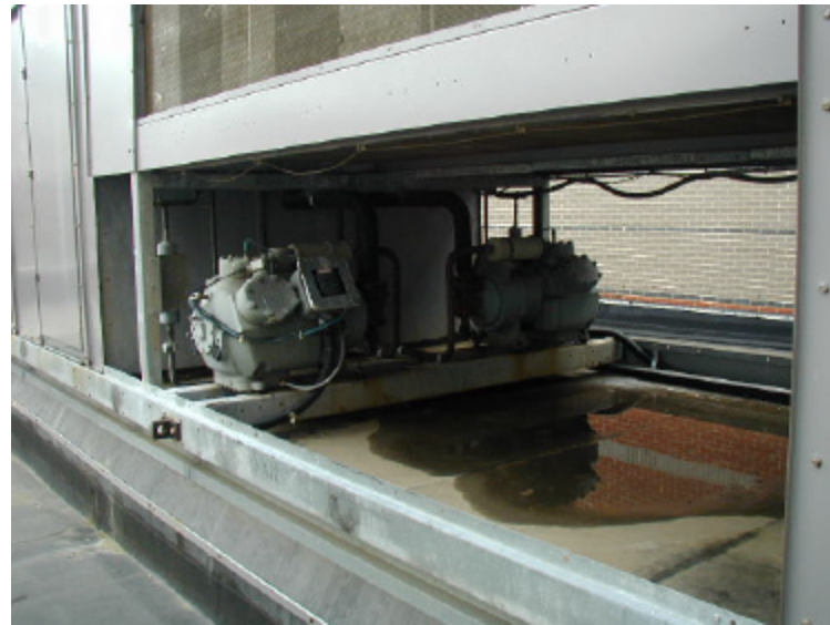
2 compressors operating in series (refrigerant charge of 73.5 and 64.5 lbs R-22)
