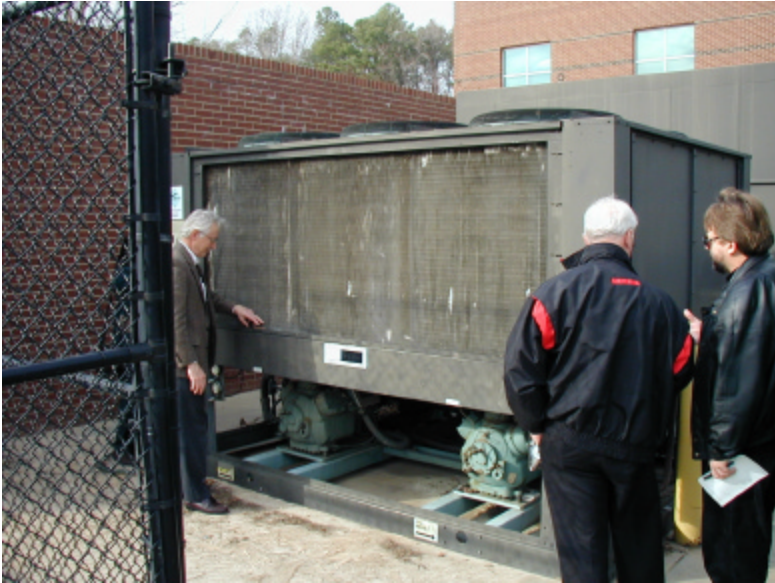
Water chiller, equipped with 2 compressors
