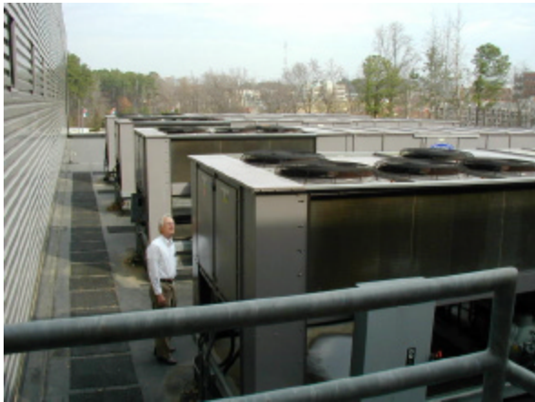
Commercial Roof-Top Air Conditioning System
