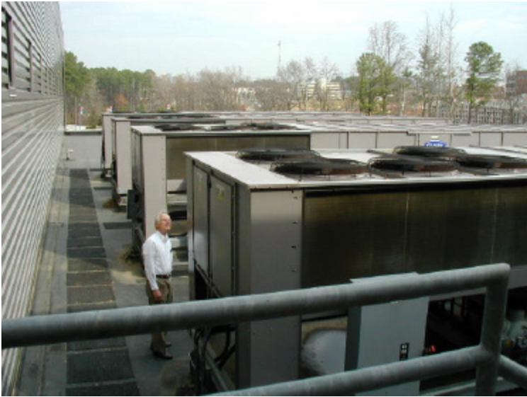
4 air conditioning systems, each equipped with 2 compressors (30 hp)
