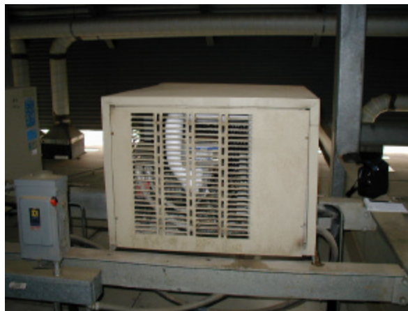
Supermarket Refrigeration System Compressor/Condenser Unit
