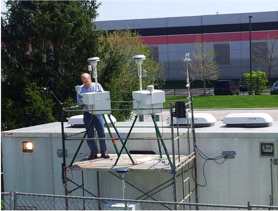
Figure 3-4. BGI PQ200 reference samplers installed at sampling site.
