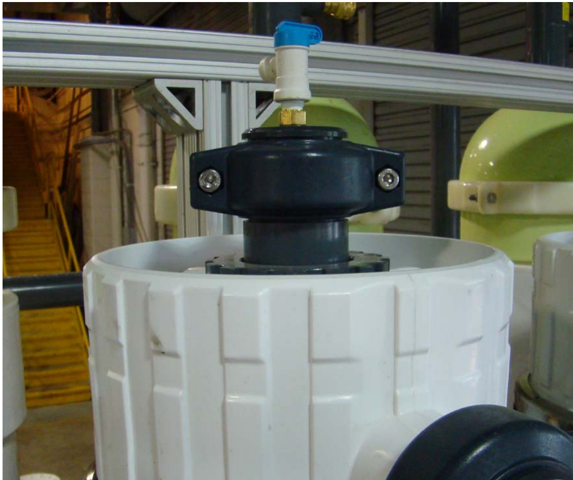
Figure 3-5. Bleed valve installed on reject port cap.
