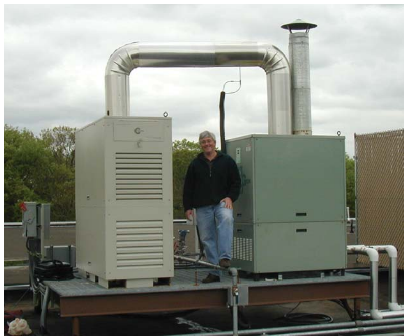
A typical microturbine CHP installation (Capstone 60 microturbine and Unifin Heat Exchanger)
