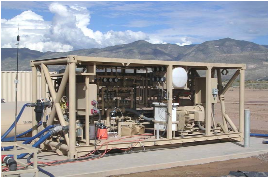
Figure 2-7. Photo of the RO skid.
