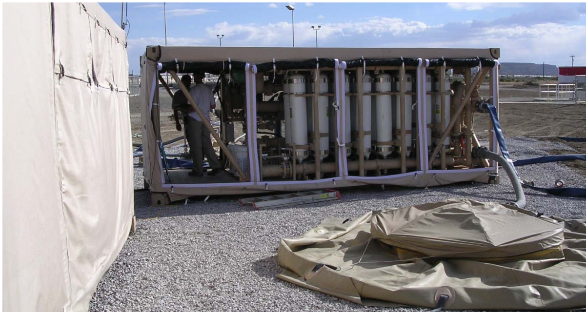
Figure 2-5. Photo of the UF skid.
