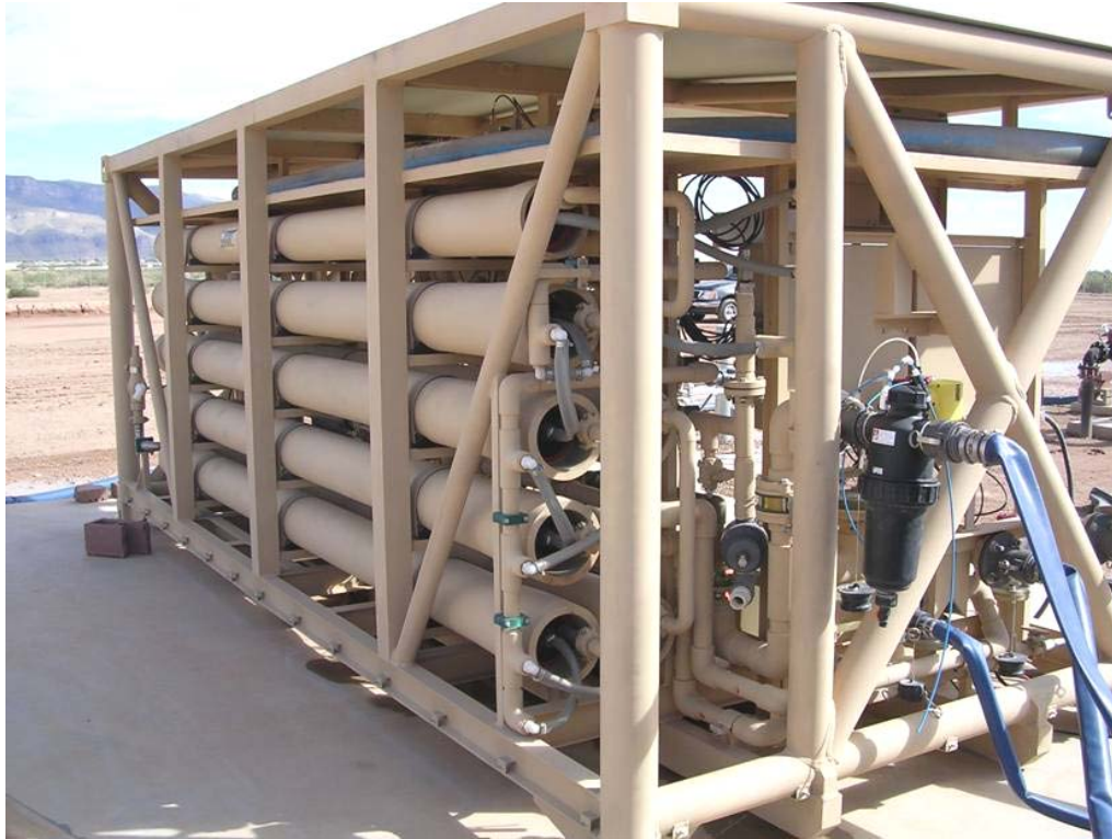
Figure 2-8. Photo of the RO skid membrane vessels.
