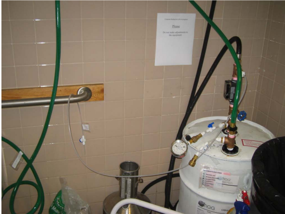
Figure 2-2. Photo #2 of the Brimac pilot unit.
