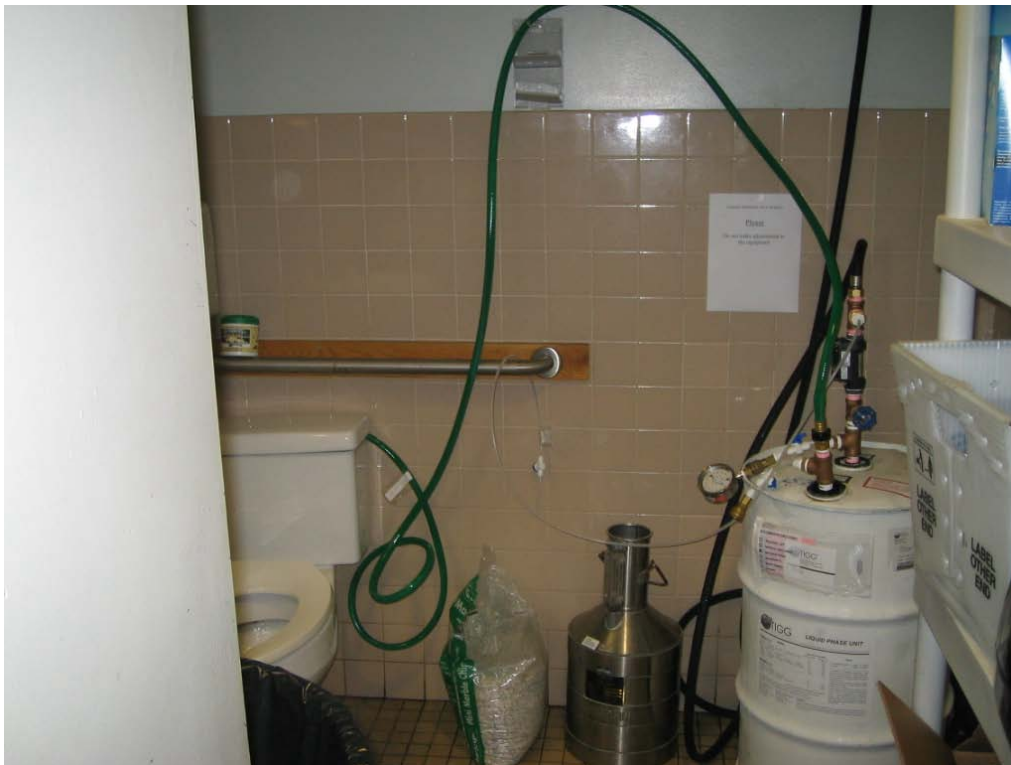
Figure 2-3. Photo #3 of the Brimac pilot unit.
