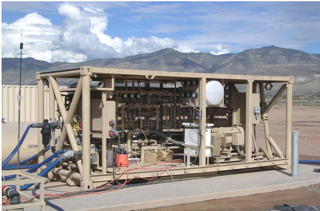
Figure 2-8. Photo of the RO skid.
