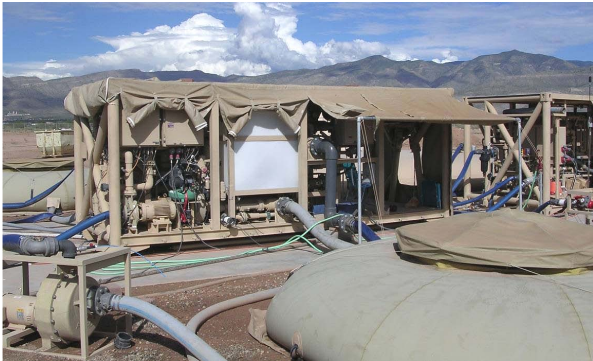
Figure 2-5. Photo of the UF skid.
