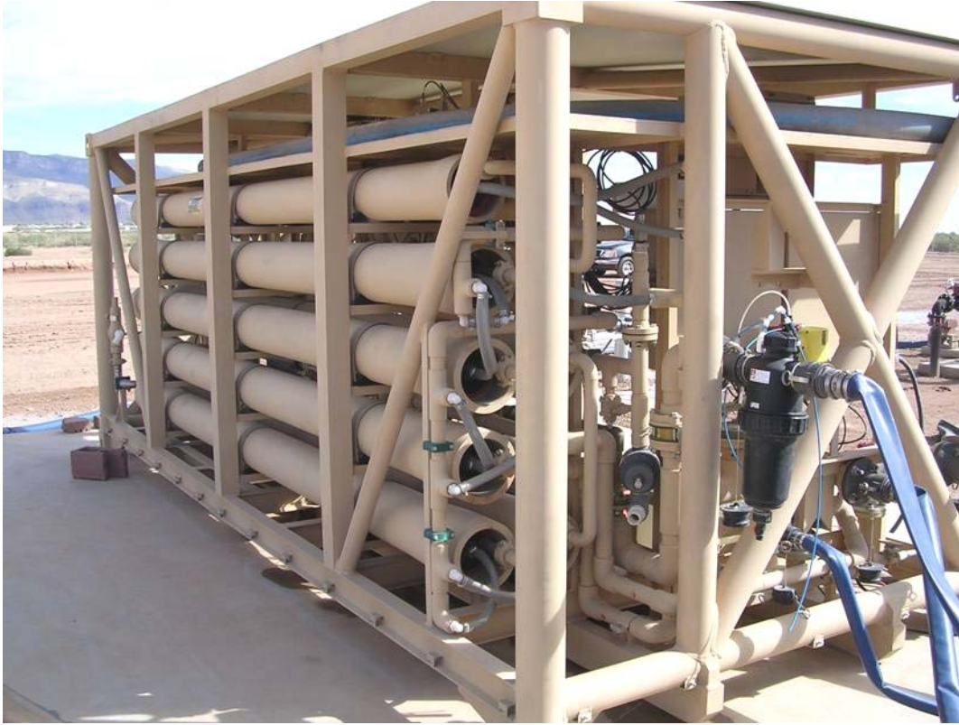
Figure 2-9. Photo of the RO skid membrane vessels.
