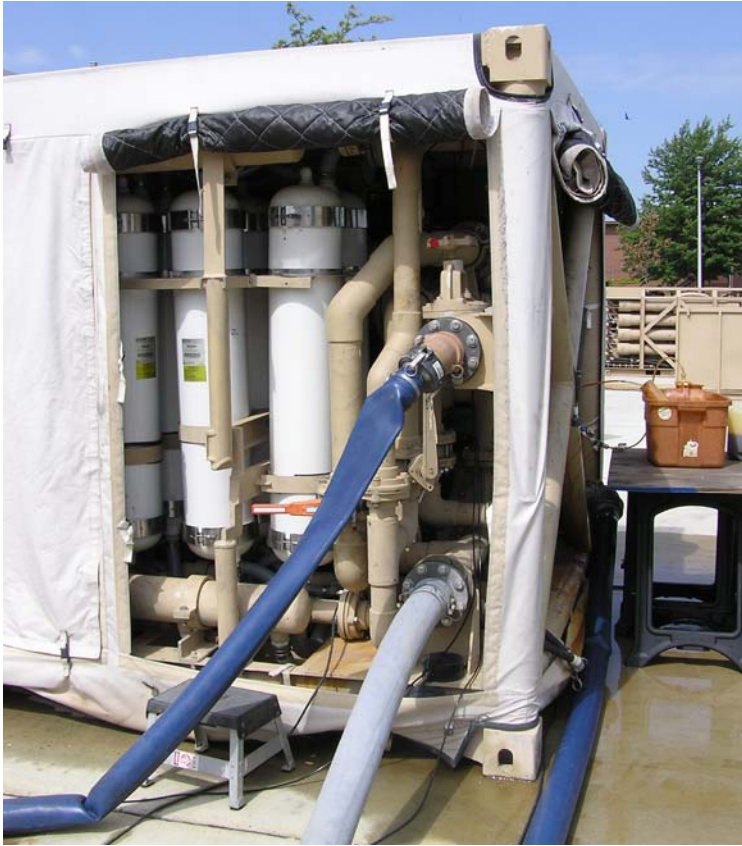
Figure 2-6. Photo of the UF cartridges mounted in the UF skid.
