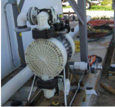
Figure 10. Yamada NDP-80 Air diaphragm pump as installed.
