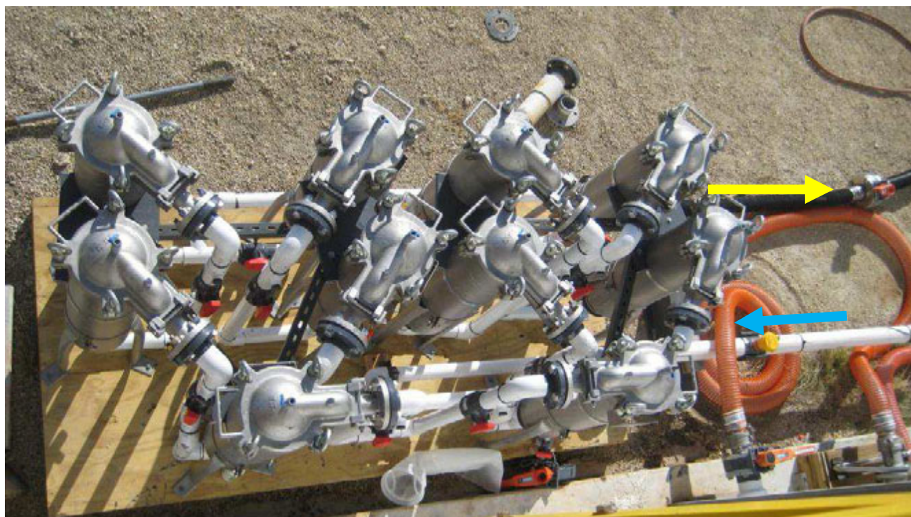
Figure 9. Plan view of the prototype filter skid at NRLKW. Blue arrow shows water entering the filter skid; yellow arrow shows water exiting the skid.
