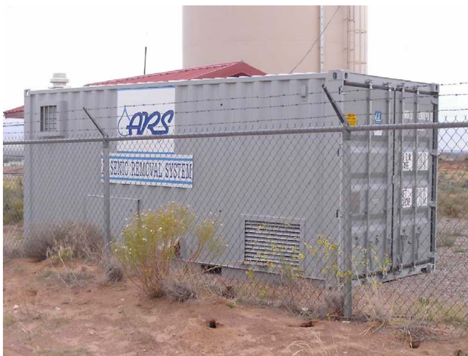
Figure 2-3. ARS CFU-50 APC skid-mounted unit photograph.
