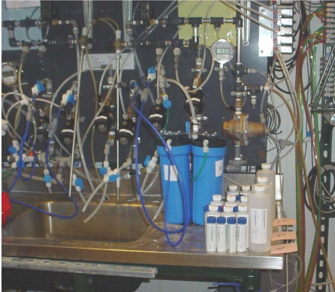
Figure 3-2. Post-Membrane Carbon Filters Installed at Test Station
