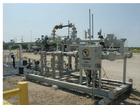
The COMM Engineering EVRU™ installed
