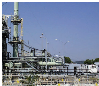
One of the test locations for mercury CEM verification
