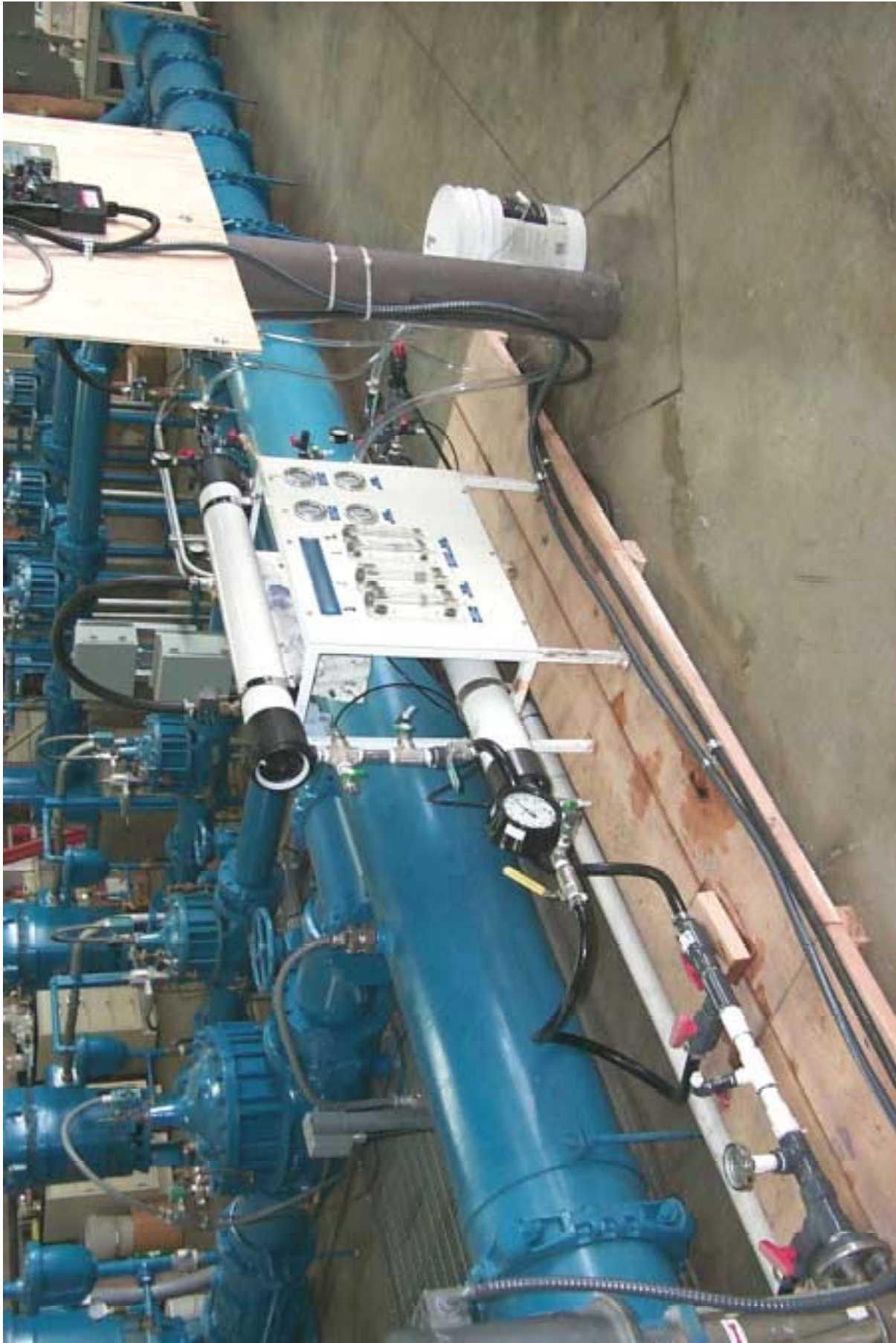
Photograph 3: Membrane Element Module Test Unit showing feed end of module
