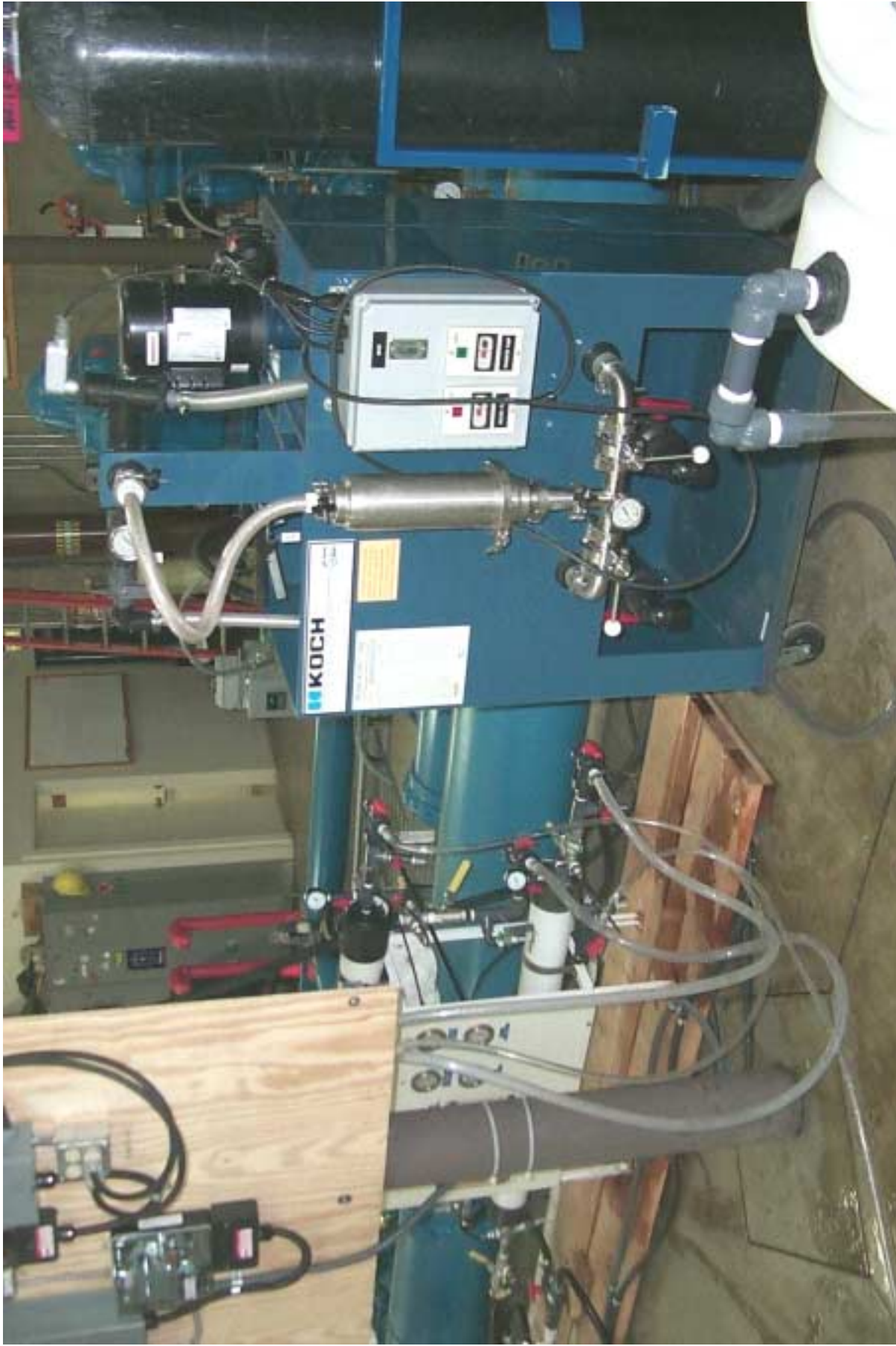
Photograph 5 – CIP unit used for cleaning membrane element modules.
