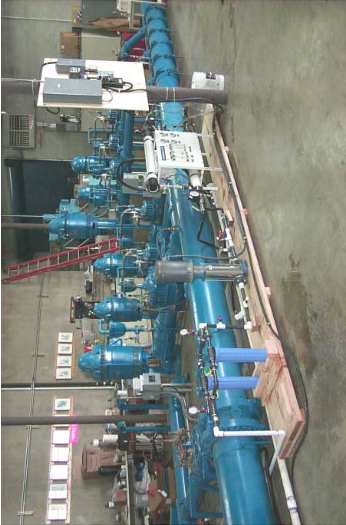
Photograph 1: Membrane Element Module Test Unit showing prefilter housing and high pressure pump
