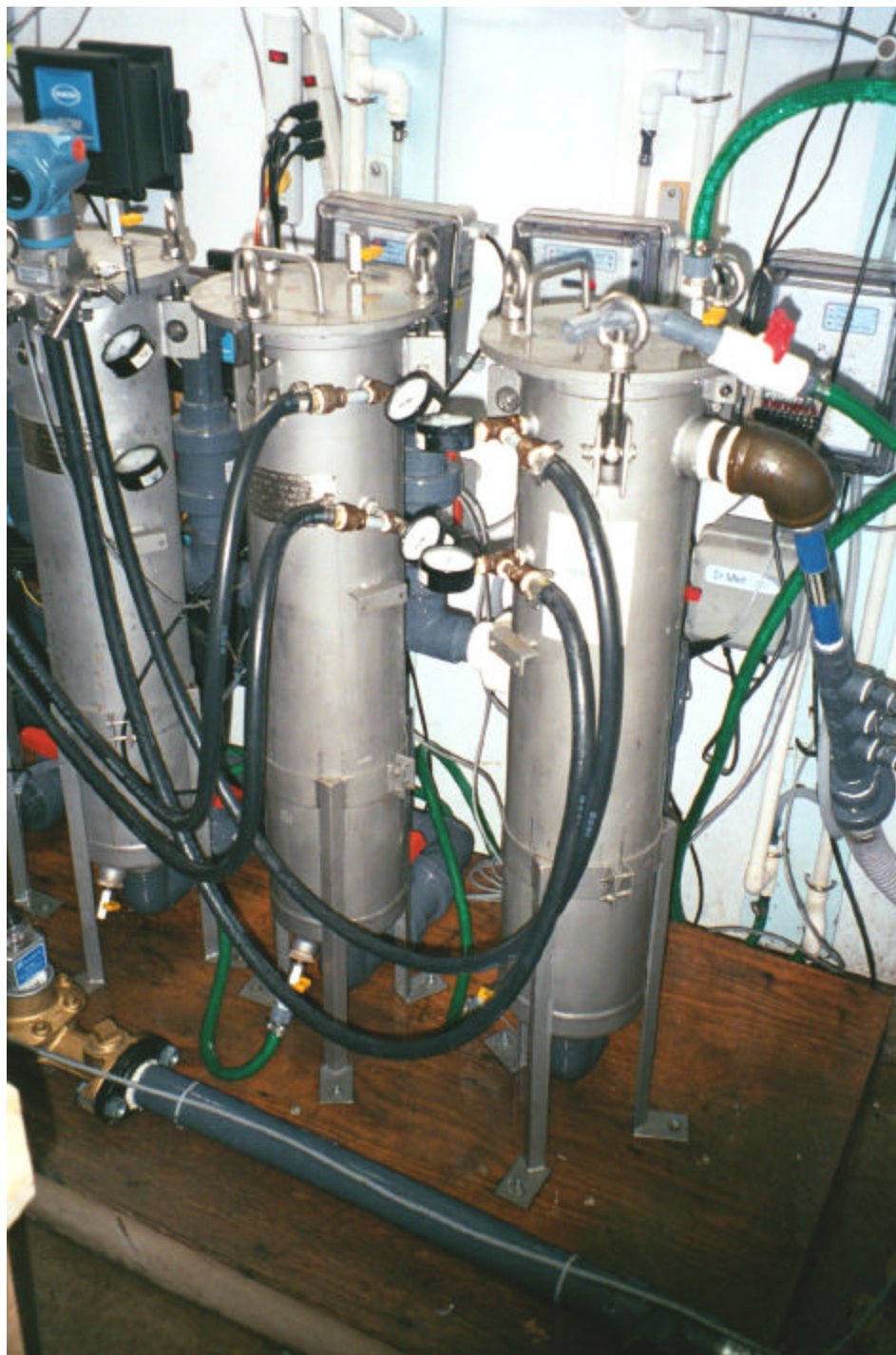
Photograph 21. Treatment System as Installed at Burnside Borough (including pressure vessels, pressure gauges and particle counters)
