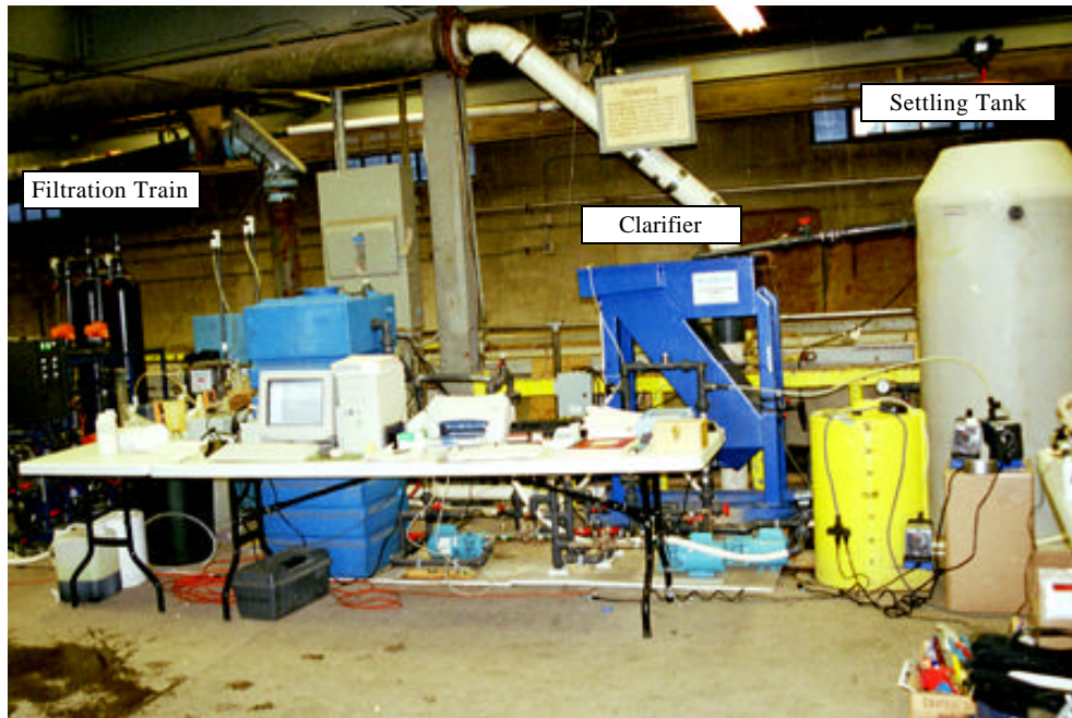
Photo 1. Front view of the Kinetico CPS100CPT Coagulation and Filtration System at SAFHL
