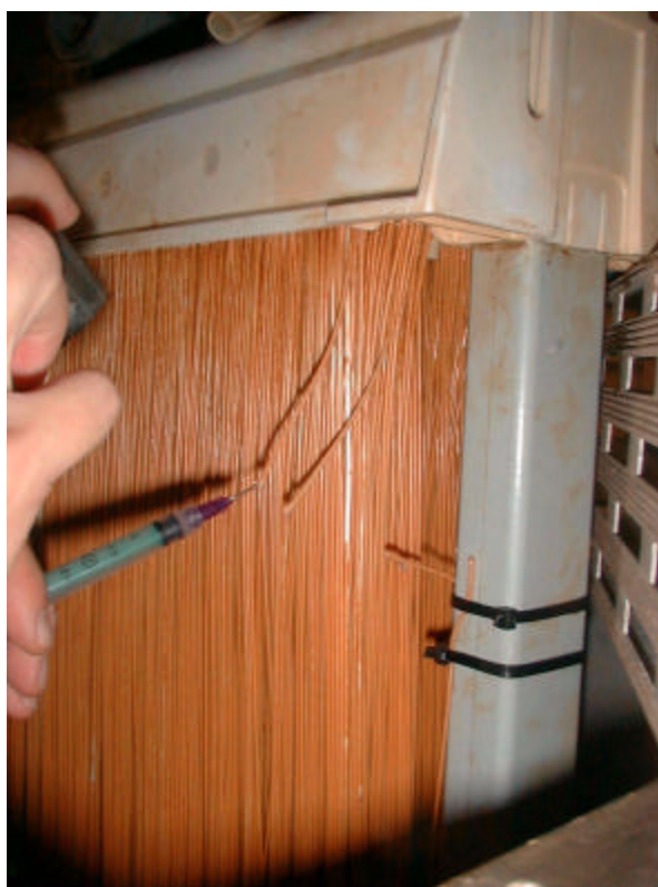
Figure 4-17. Seal Repair of Damaged Fiber with Epoxy
