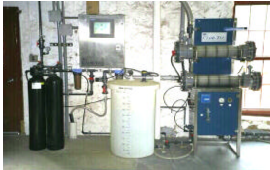
Photograph 2.2 Softener, PLC, Brine Day Tank and Hypochlorite Generator
