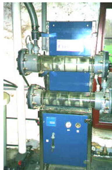
Photograph 2.3 Sodium Hypochlorite Generator
