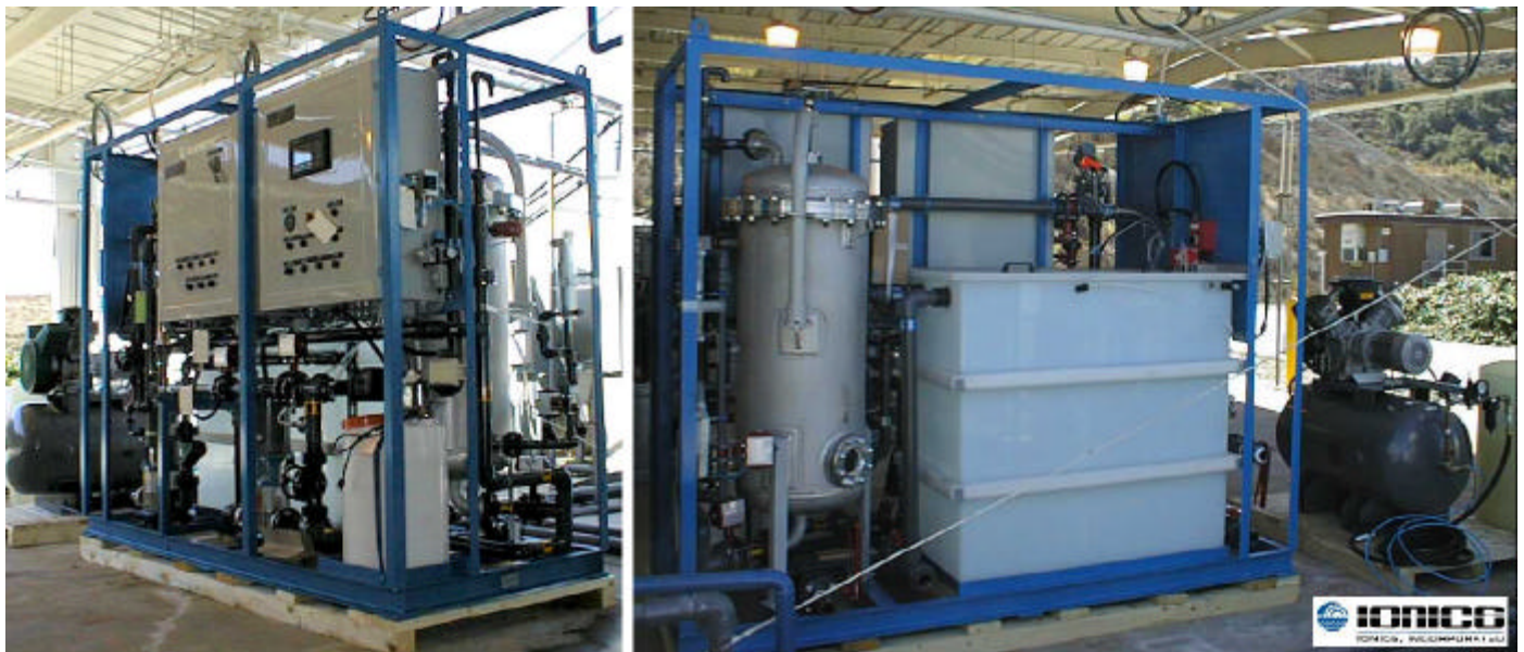
Figure 2-1. Photographs of ETV test unit.
