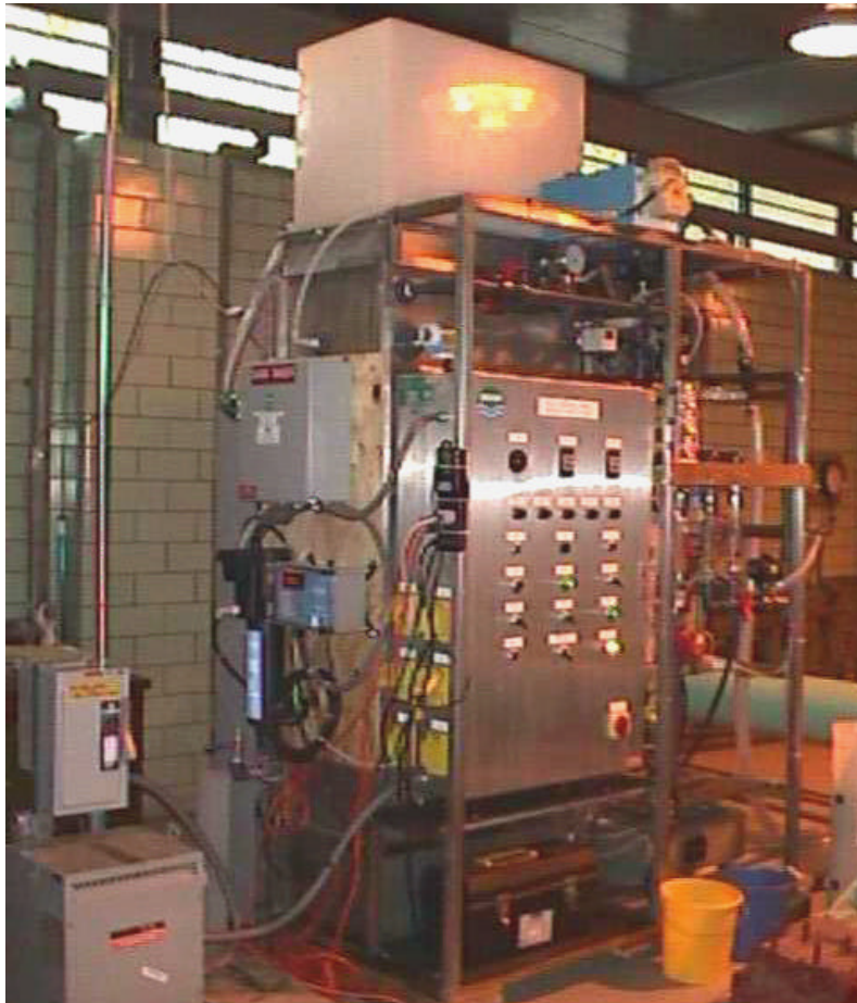
Photograph 1. The ZENON Environmental Inc. ZeeWeed® ZW-500 UF Drinking Water System showing control panel, process tank, bleed pump and ancillary equipment.
