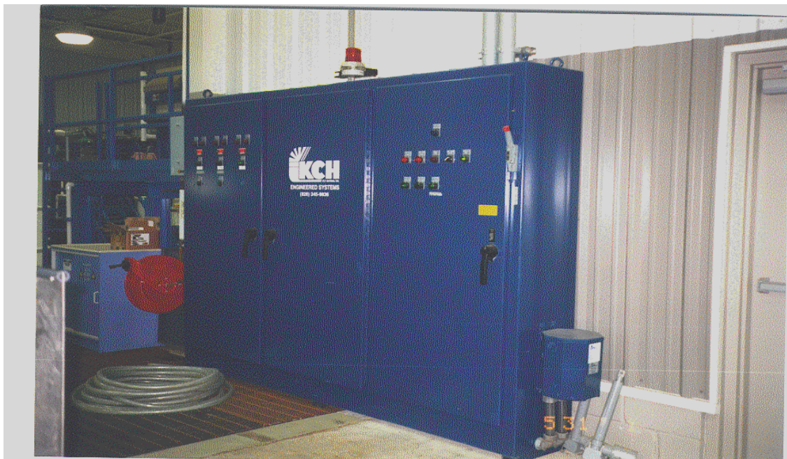
Figure 4. KCH ACTSEC Electrical Control Cabinet
