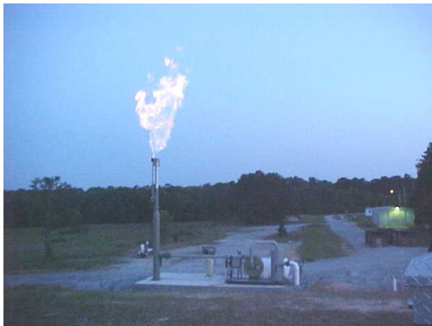
Figure 3: Collection System & Flare (subsequently fenced)
