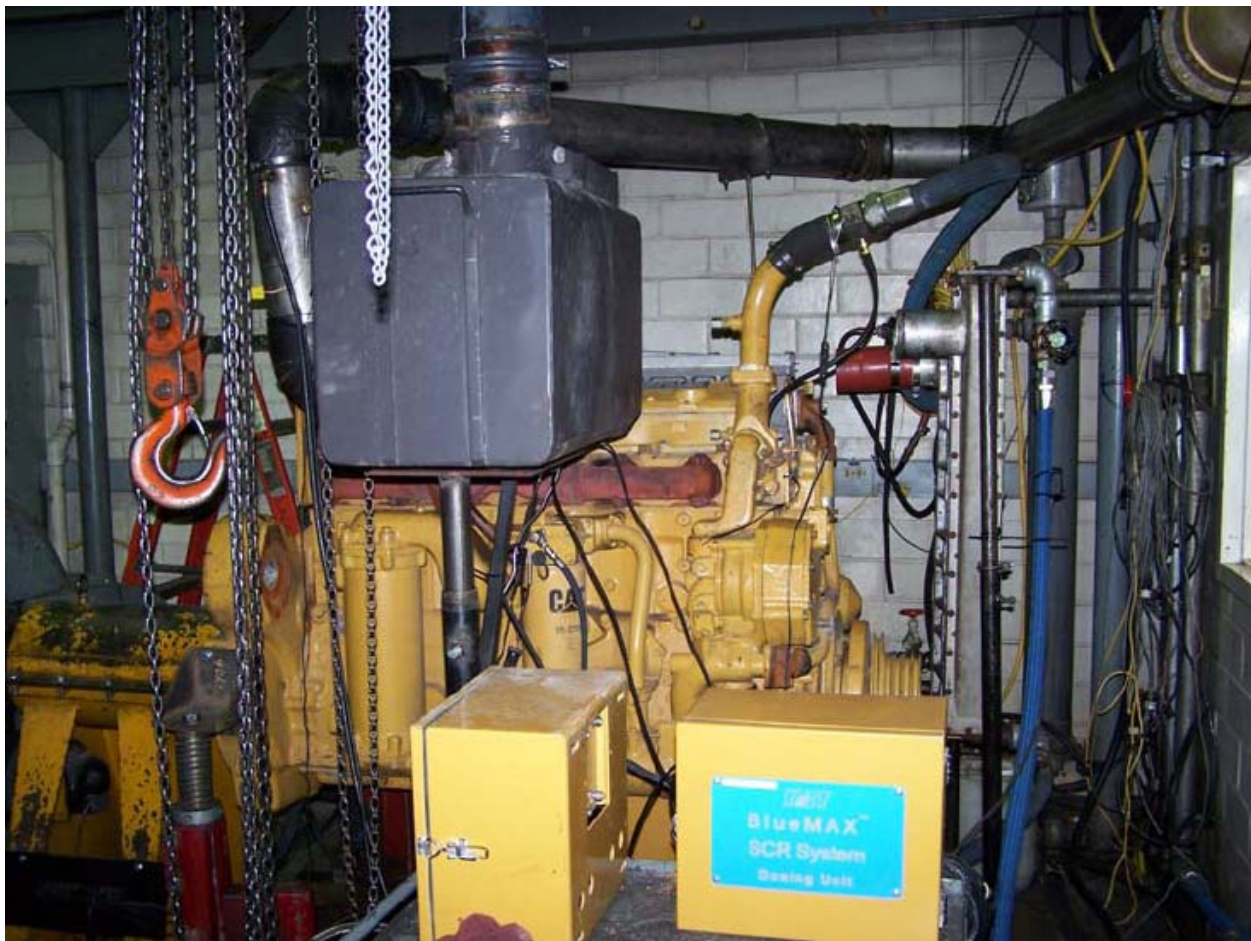
Figure 1. The BlueMAX 100 Version A Urea-Based Selective Catalytic Reduction System installed for emissions tests.
