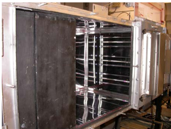
Figure 2-1. Ballast box installed on the outside of the test rig (on right). The device is also visible.
