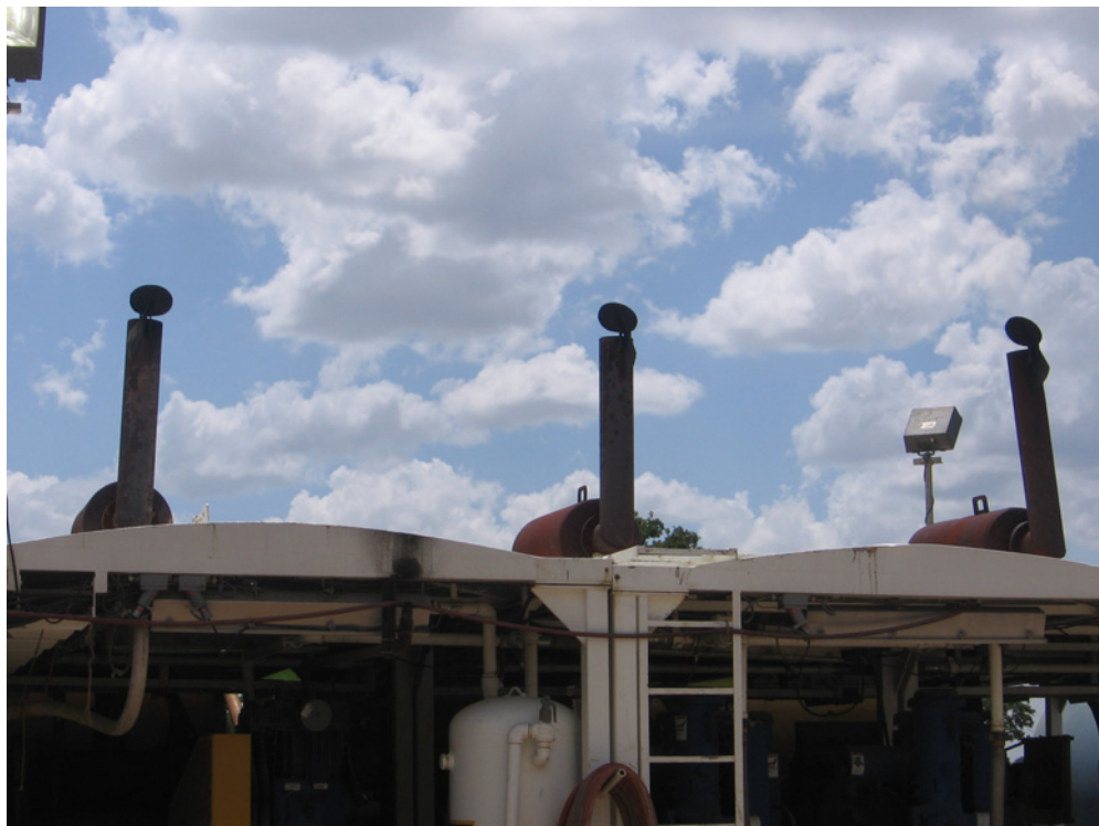
Figure 2-2. Engine Exhaust Pipes
