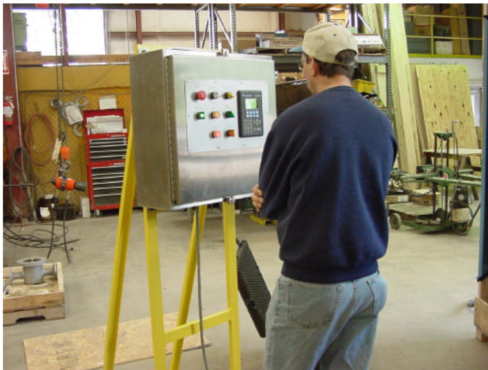
Figure 3-2. TS-5000 control panel.
