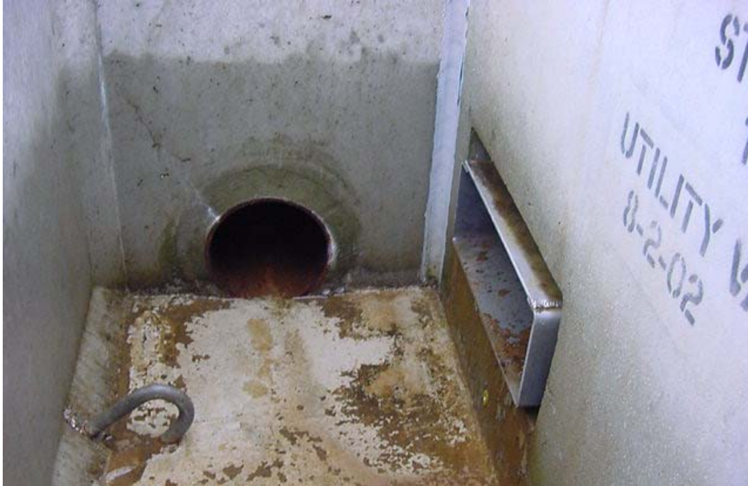
Figure 7-3. Effluent bay of StormScreen testing vault, showing rectangular discharge flume and 8-in return pipe to reservoir.
