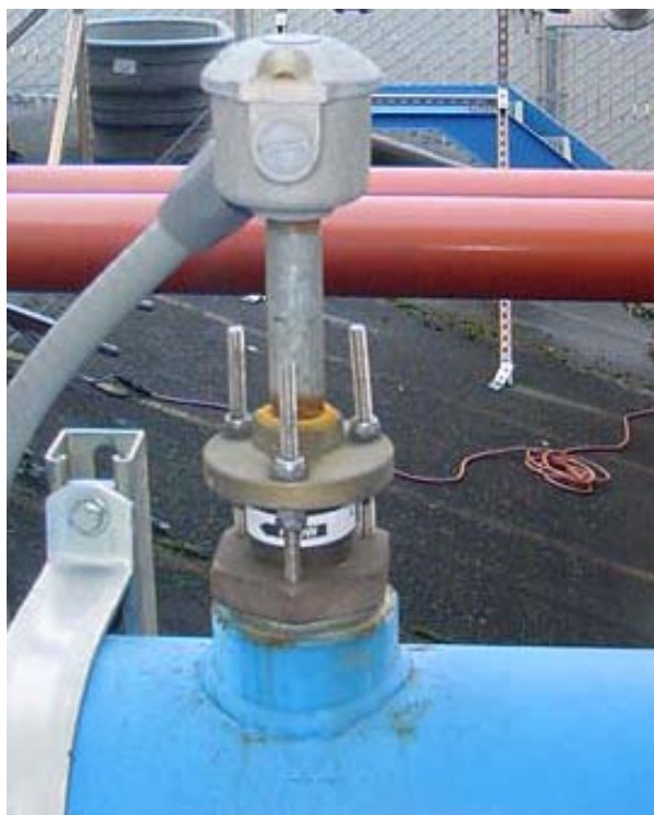
Figure 7-2. Electrically actuated control valve and in-line flowmeter.
