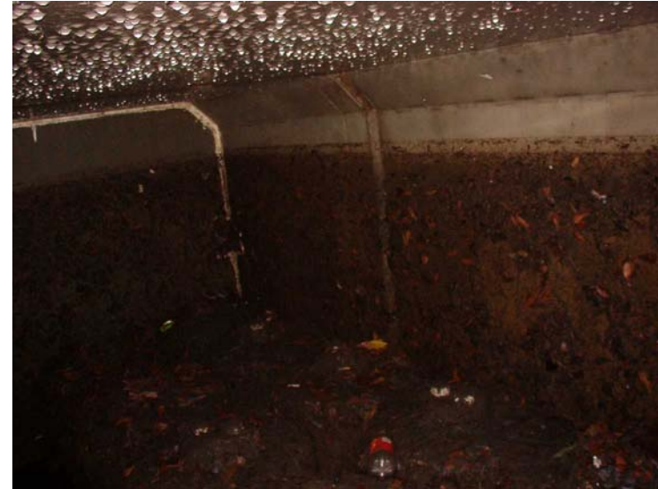
(b) StormScreen vault, November 5, 2003
