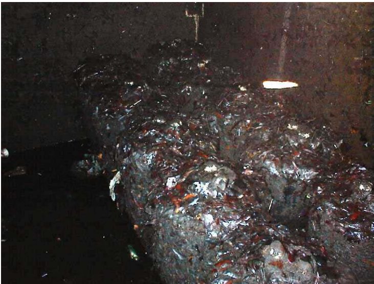
(c) StormScreen vault, January 17, 2004
