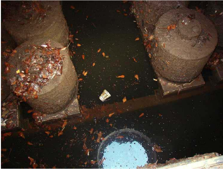
(a) StormScreen vault, November 5, 2003
