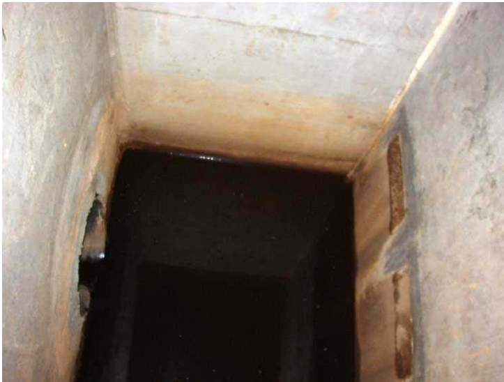
(c) StormScreen outlet bay, October 26, 2003
