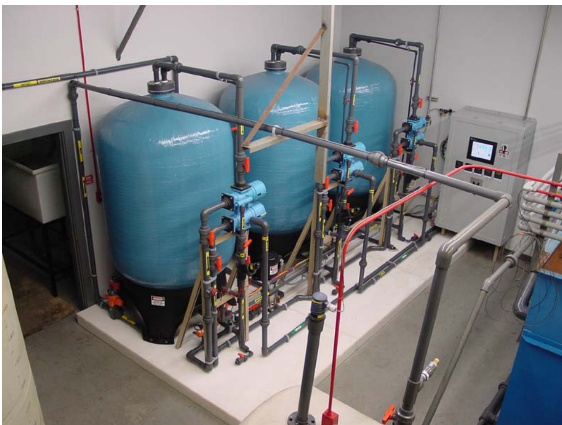
Figure 6. Photograph of the Ion Exchange System Installed at Gull Industries
