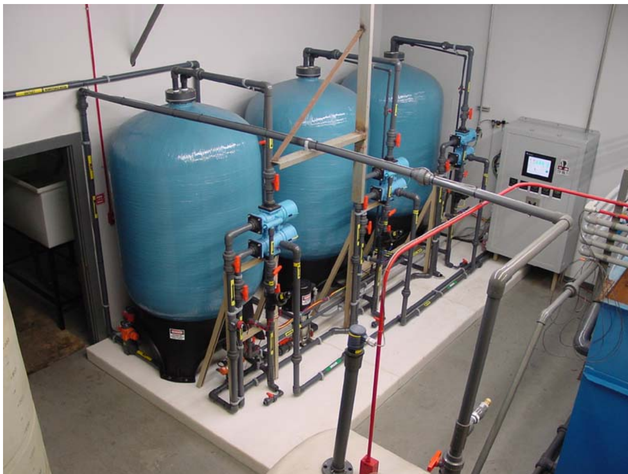
Figure 6. Photograph of the Ion Exchange Polishing System Installed at Gull Industries
