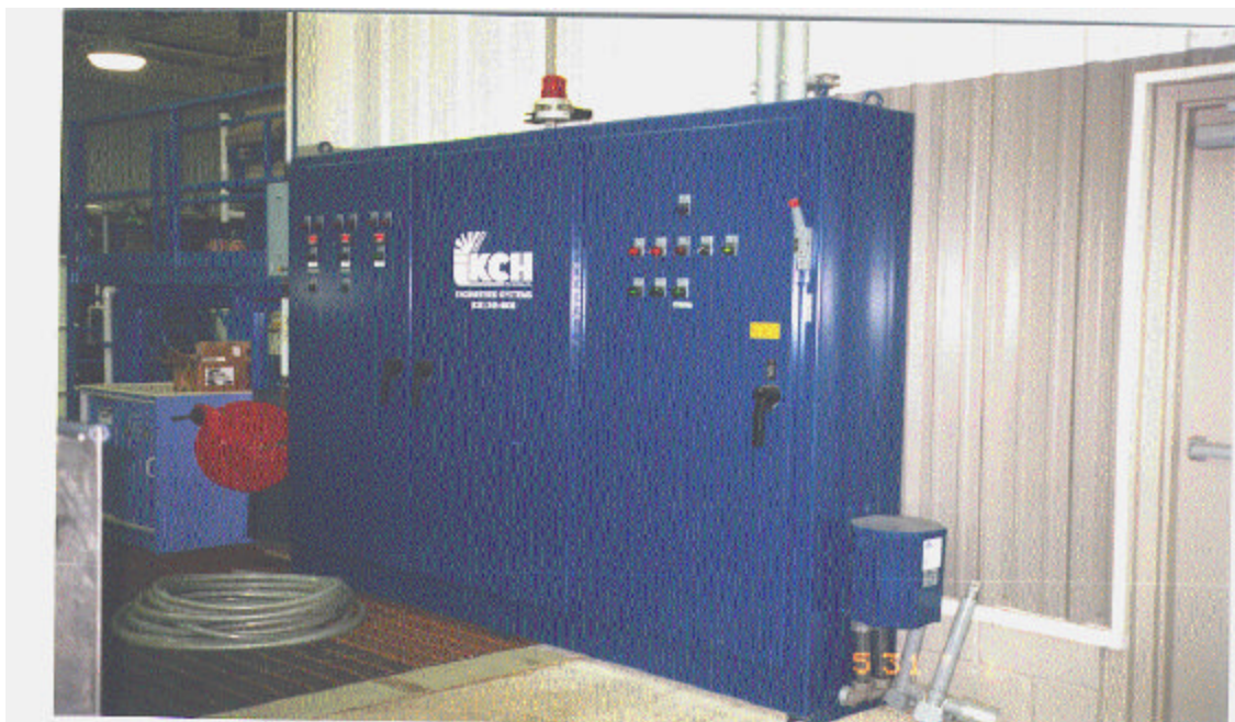
Figure 6. KCH ACTSEC Electrical Control Cabinet
