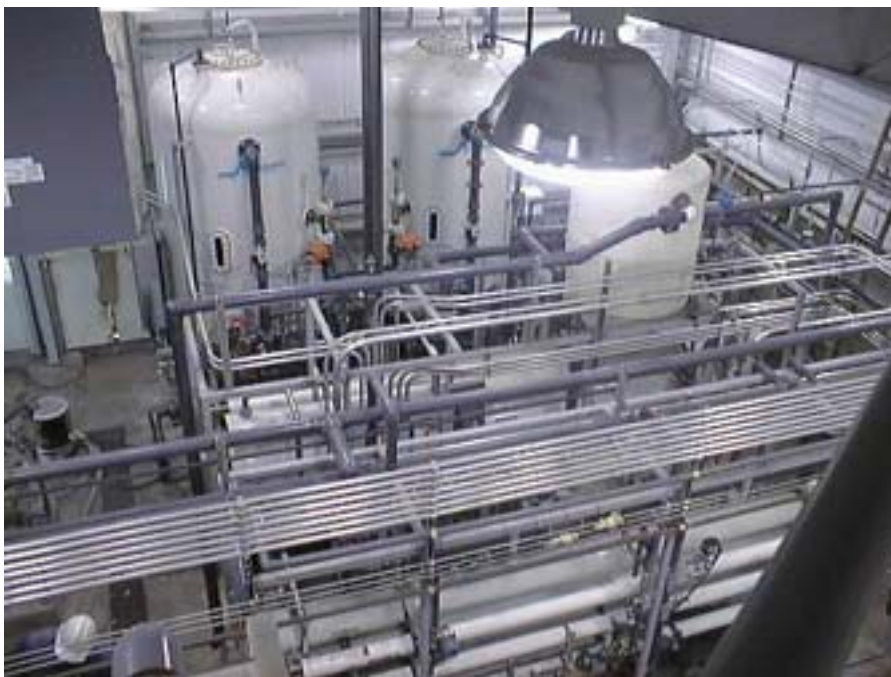
Figure 3: HERO™ Wastewater Treatment System
