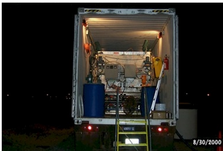
Figure 2. Interior of DTIC IWTP-MF System
