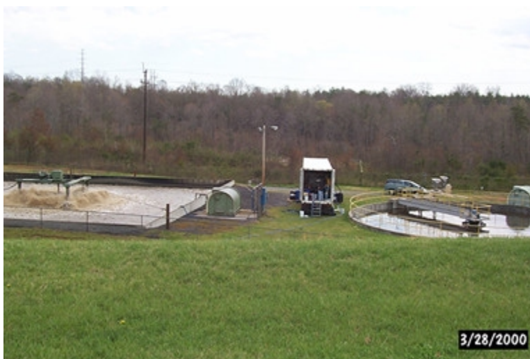
Figure 4. DTIC IWTP-MF in Use at an Industrial Site
