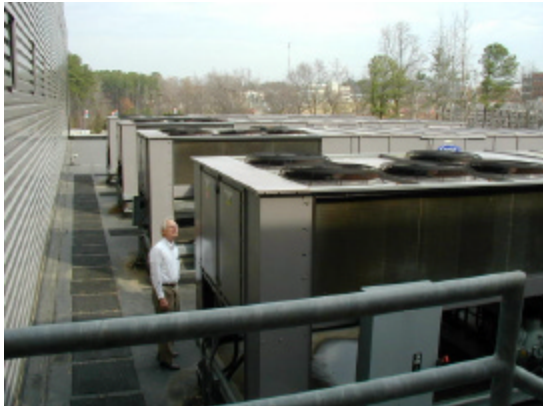
Commercial Roof-Top Air-Conditioning System
