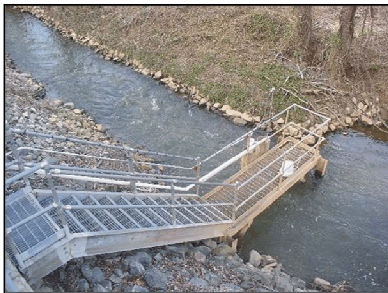
Figure 3-2. DuPont Spruance Final Effluent
