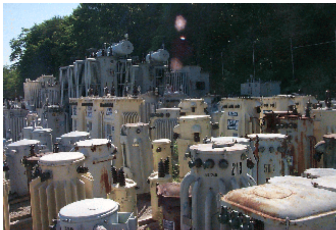
Figure 5-3. Transformer yard at ORNL.
