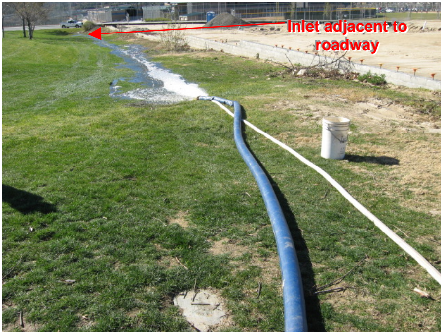
Photograph 14: Non-potable reclaimed water was pumped to a grass drainage swale and subsequent storm drain inlet leading to the Pechanga Parkway Drainage Channel
