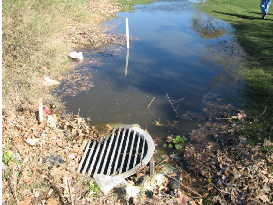
Photograph 15: View of discolored discharge to a down-gradient storm drain inlet
