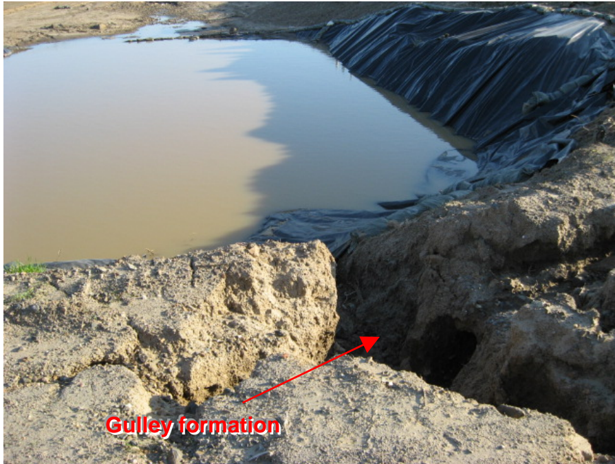
Photograph 5: Sediment laden water in the structural control and gulley erosion present at the inlet area
