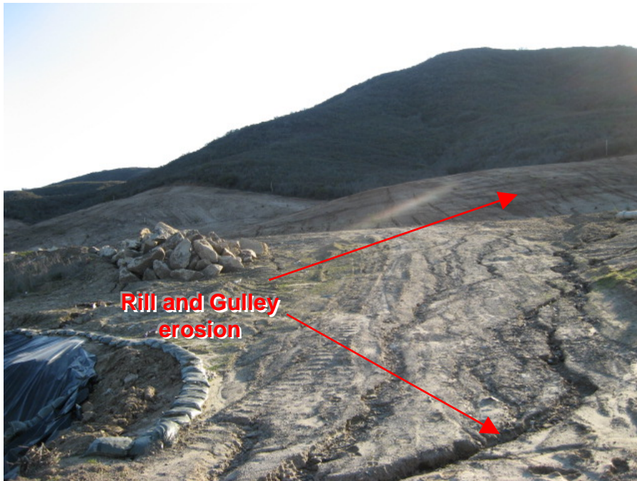
Photograph 6: Rill and gulley formations on the disturbed slope leading to the sediment trap BMP
