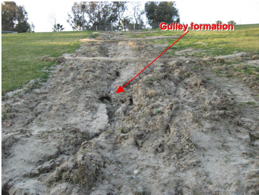
Photograph 2: Slope erosion was observed, including rill and gulley formation at the base of the slope
