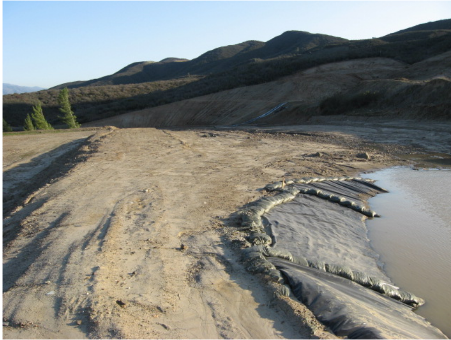
Photograph 7: A large area of exposed soil was observed down-gradient of the sediment trap BMP
