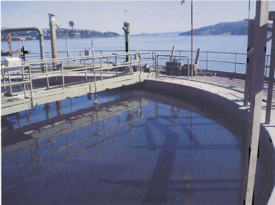
Figure 3: Primary clarifier. Note covered weir.
