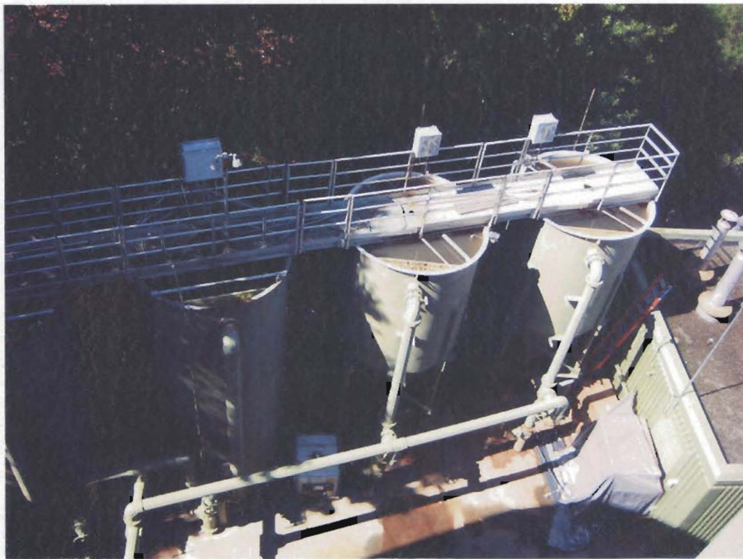
Figure 6: Sand filters. Photo taken from top of FFRs.
