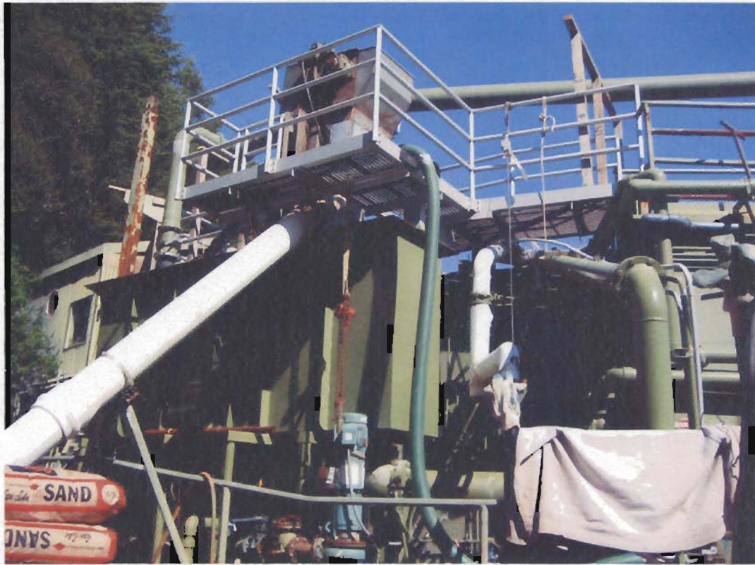
Figure 11: Grit removal at primary clarifier.
