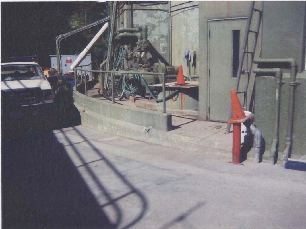
Figure 13: Digester located beneath primary clarifier.
