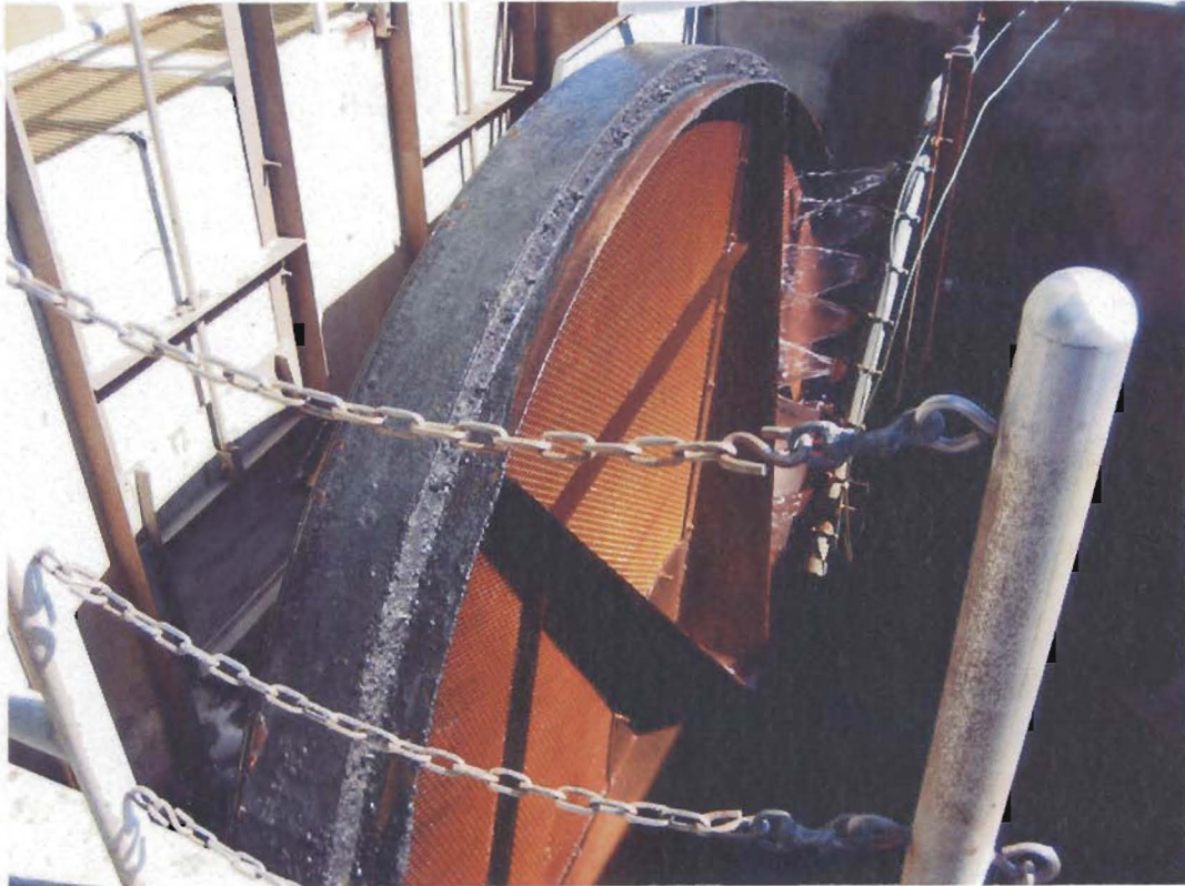
Figure 7: Secondary effluent passes through rotating screen.
