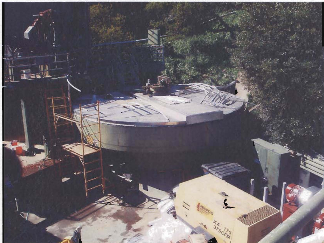
Figure 12: Gravity thickener tank.
