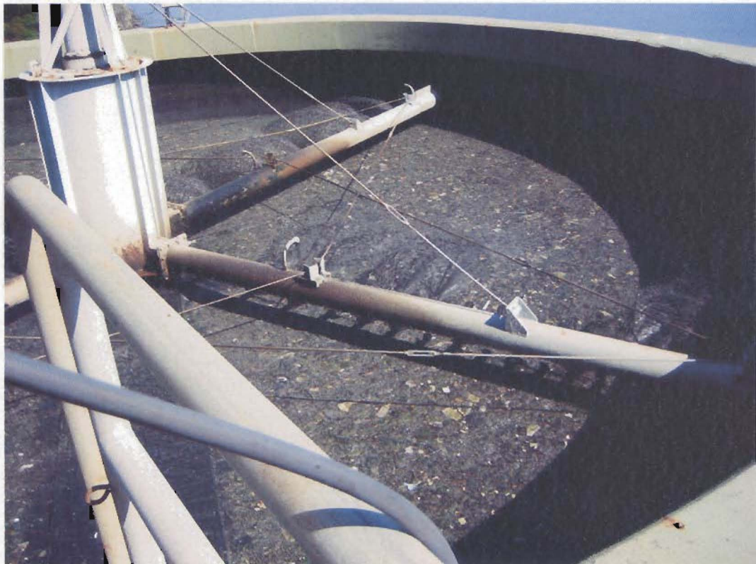
Figure 4: FFR #2. Note extensive debris on screen and debris-clogged nozzles.
