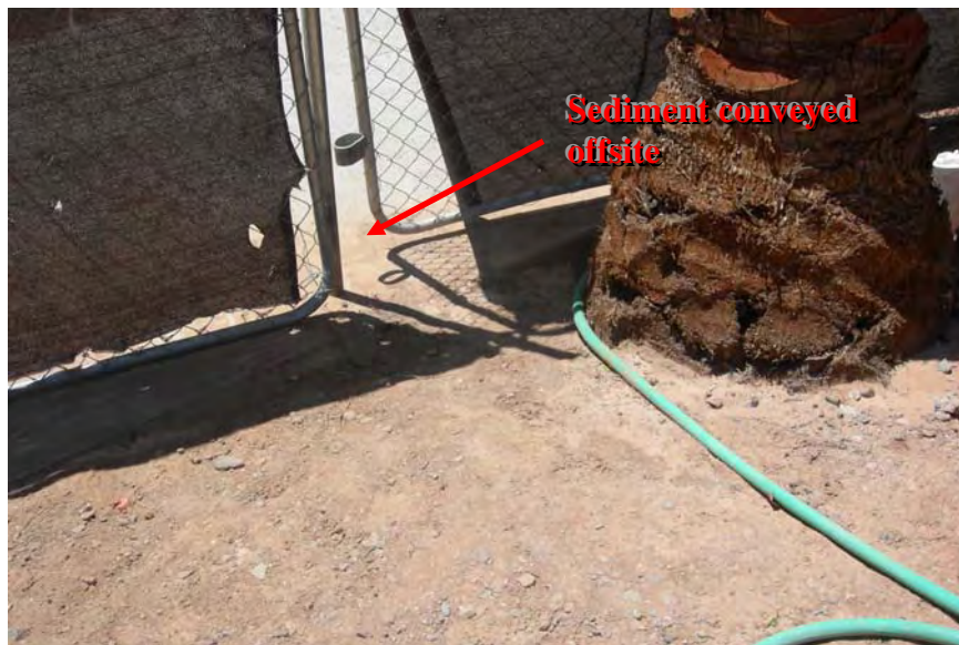
Photograph 6. View of sediment release along the east side of the Scottsdale Fashion Square construction site, adjacent to Scottsdale Road.
