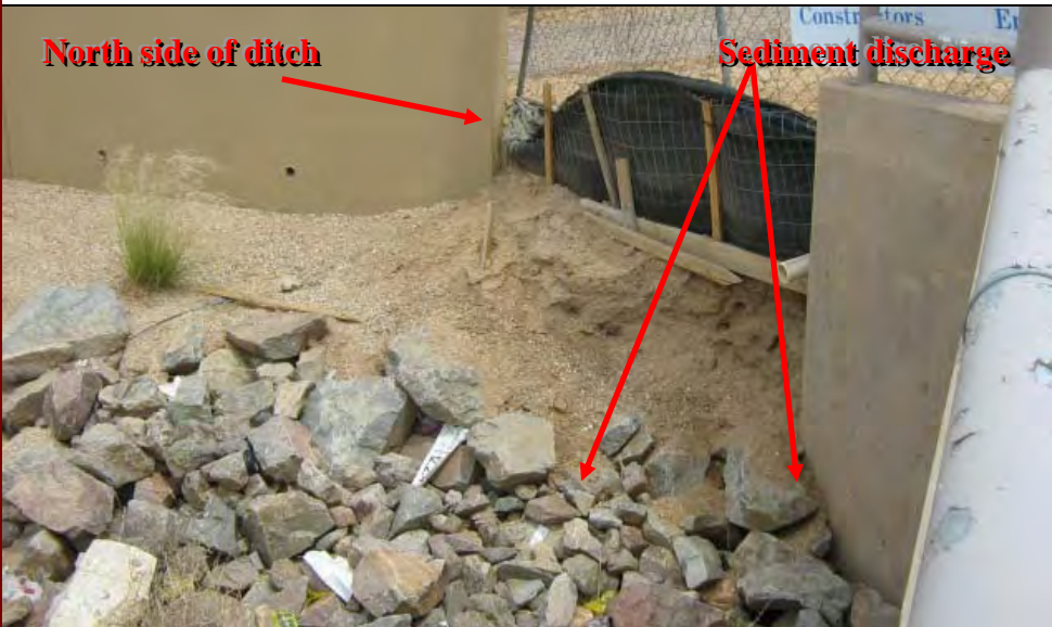
Photograph 7 – Silt fence failure and offsite sediment
