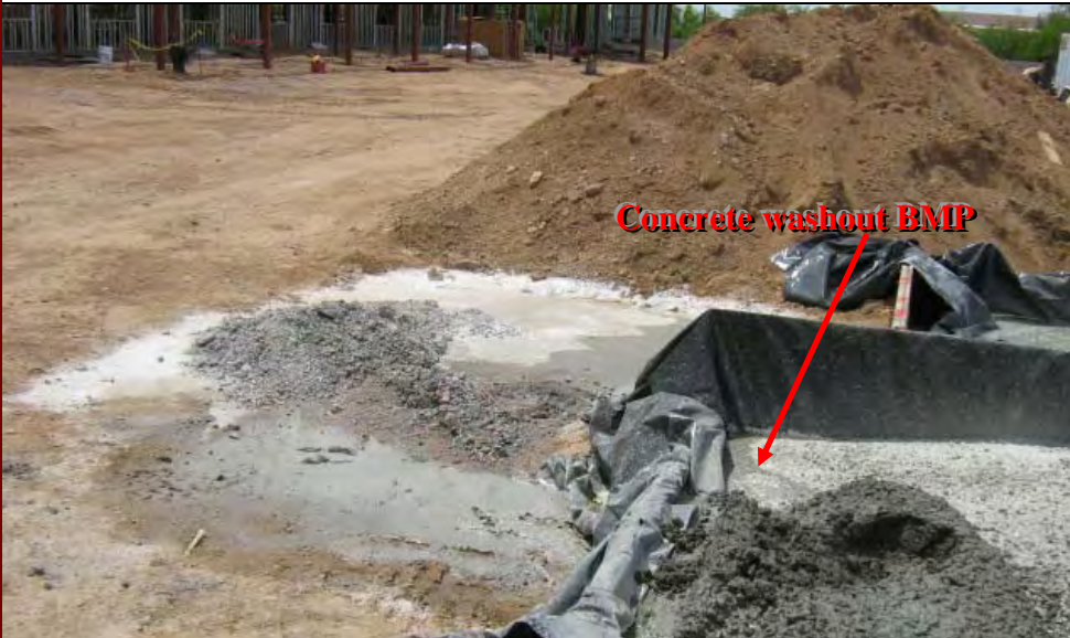
Photograph 5 – Concrete waste beyond the dedicated concrete washout BMP
