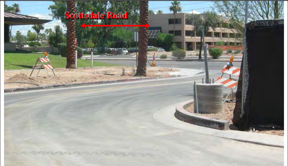
Photograph 4 – View of sediment tracking at the construction entrance at the northeast corner of the site.
