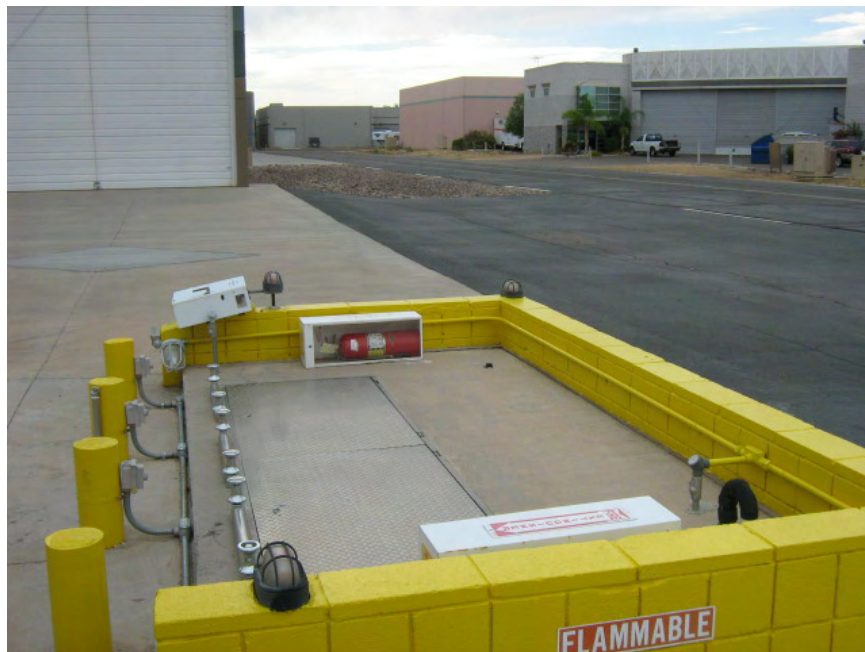
Photograph 4. Scottsdale Airpark – Aircraft fueling system located northeast of 7916 East Beck Lane in Scottsdale, Arizona
