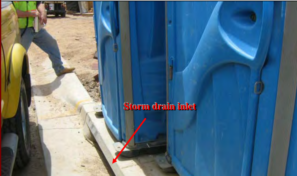
Photograph 11 – Portable toilet improperly placed directly adjacent to inlet
