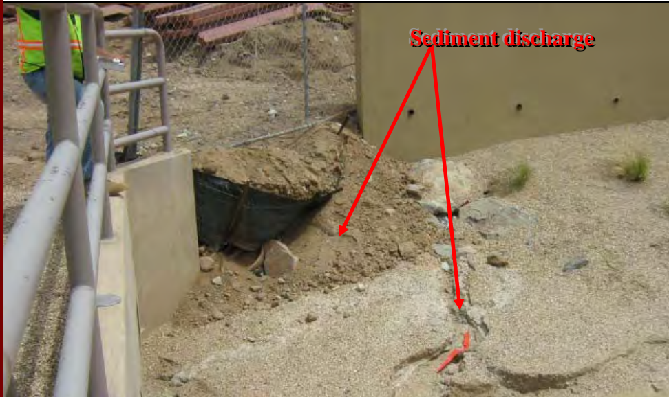
Photograph 9 – Silt fence failure and offsite sediment
