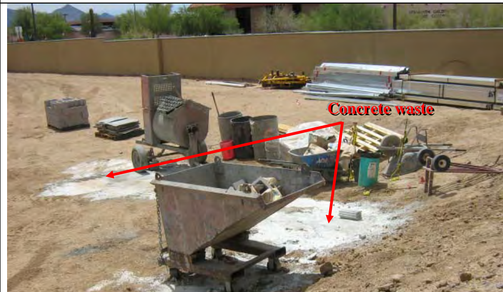
Photograph 4 – Potential source of the illicit discharge
