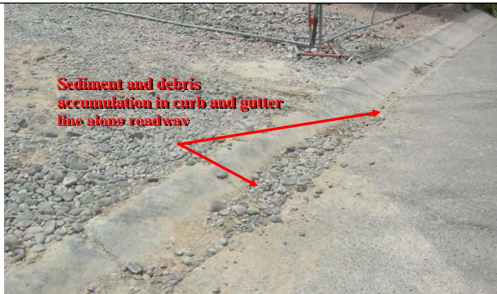
Photograph 4 – Sediment and debris accumulation at Phase II construction entrance
