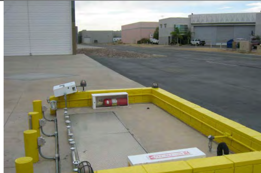
Photograph 1— Aircraft fueling system located northeast of 7916 East Beck Lane in Scottsdale, Arizona
