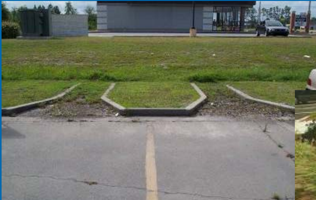
Parking lot drains to swale
