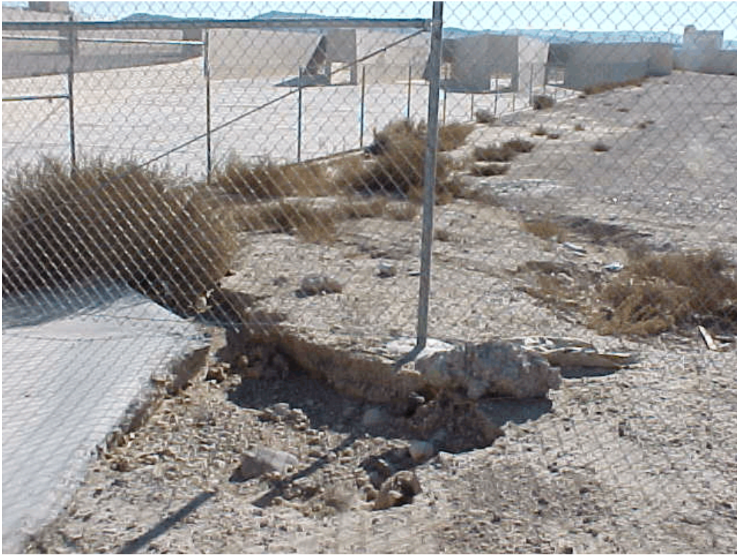
Photo 1. Erosion to the detention basin at the northeast corner.
