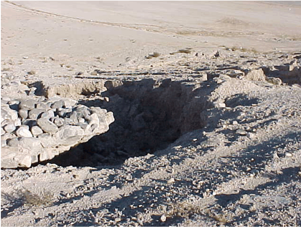
Photo 9. Erosion on west wall of detention basin.
