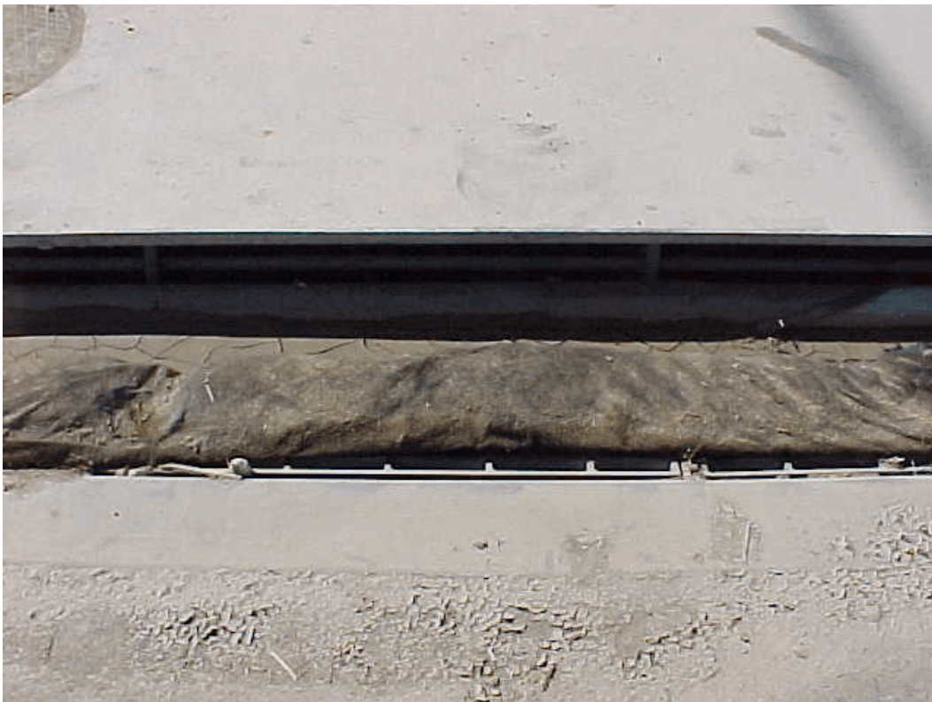
Photo 2. Street inlet protection that is poorly maintained by Landtec LLC.
