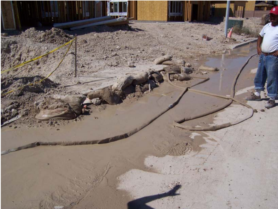
Photo 2. Storm inlet at the site. Sediment is also entering the storm sewer through the pick hole in the manhole in front of the inlet. Hose in the photo is the fire hose the site had been using to clean the street. Note poor condition of sand bags used for inlet protection and dirt extending past curb line.
