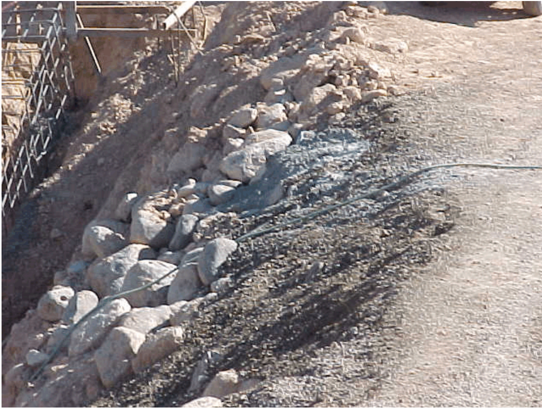
Photo 3. Closeup view of concrete washout on downstream face of earthen dam. A sump is located at the toe of the dam face (photo left).
