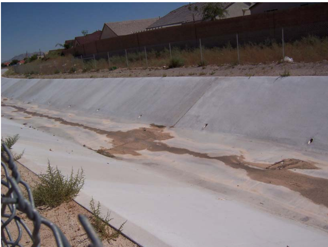
Photo 2. Wash adjacent to the construction site. Wash appears to contain sediment that may have come from the site.
