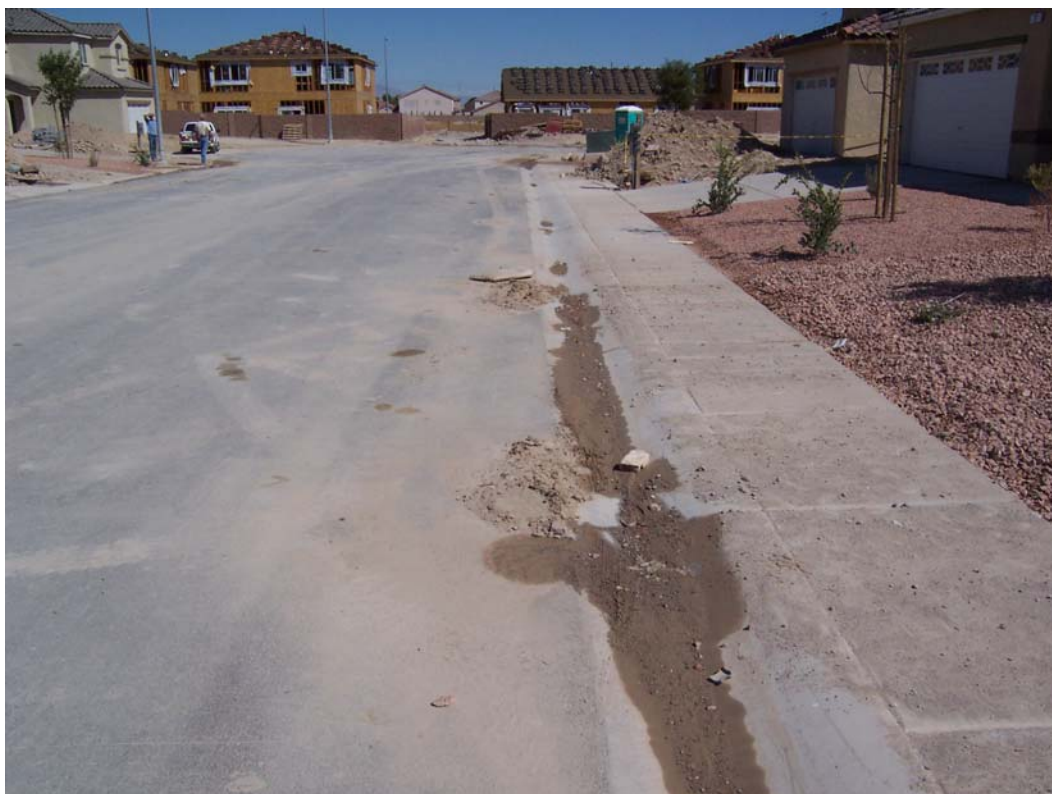
Photo 5. Sediment in the street. Moisture indicates street was washed earlier in the day. Note sand bag, center rear of photo, pulled back from the curb.
