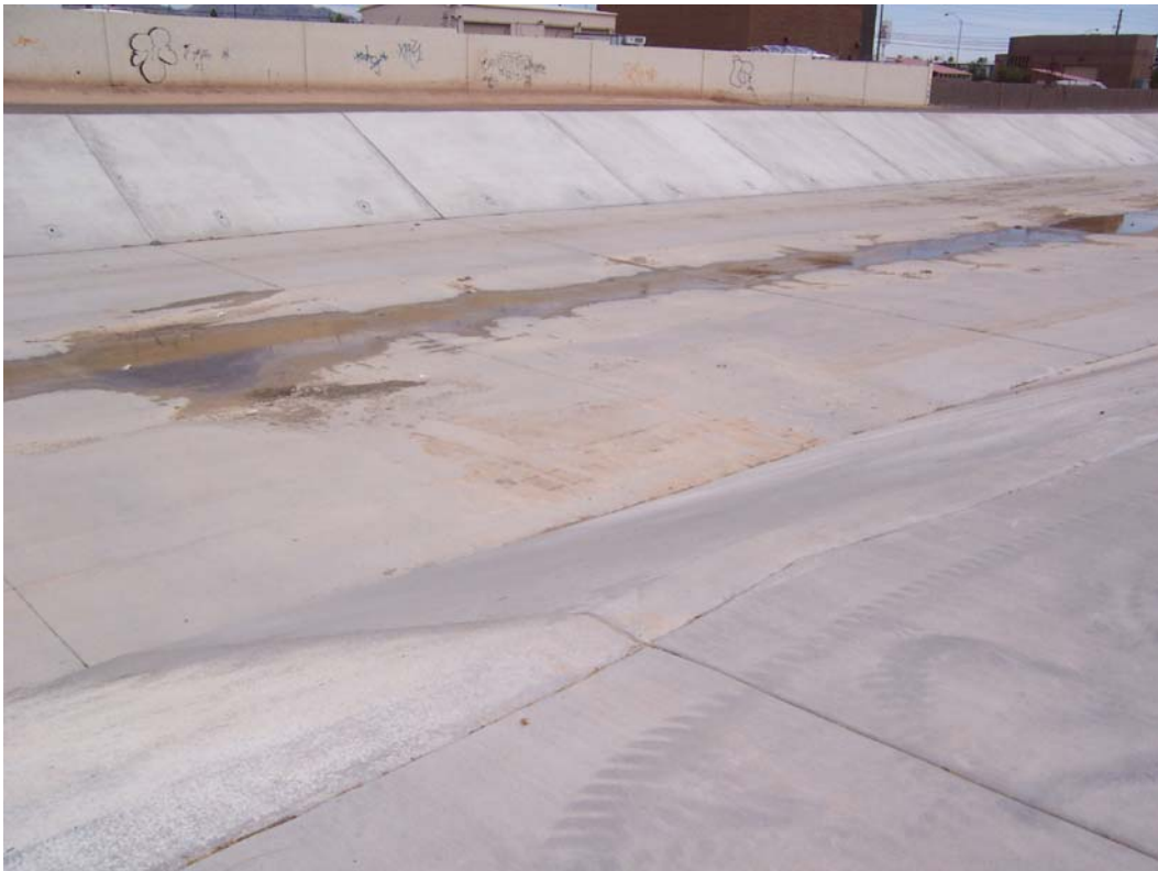
Photo 5. Portion of wash adjacent to the channel in Photo 4 where sediment appears to have entered the wash from the channel.
