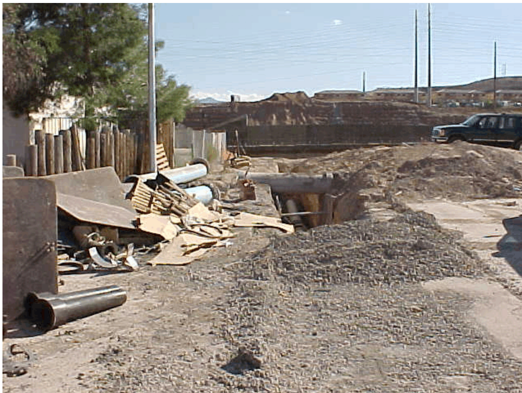
Photo 7. Additional staging area. Note uncontained five-gallon gas can (photo center).
