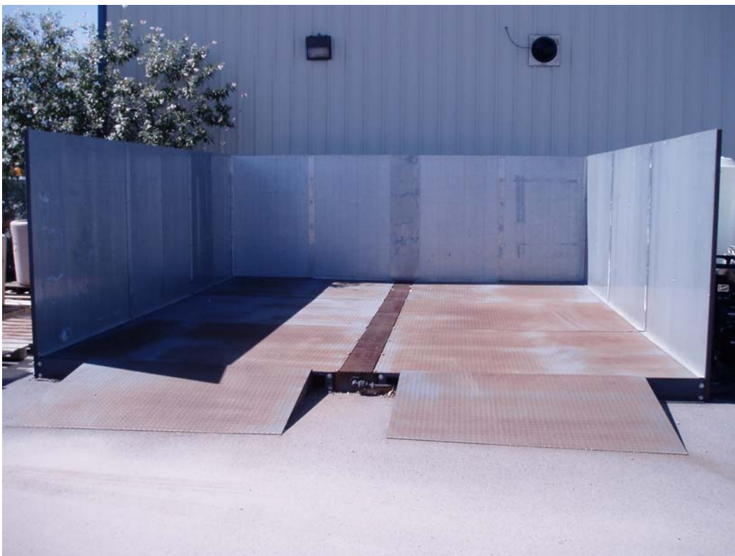
Photo 2. Equipment wash area with water recycling unit.
