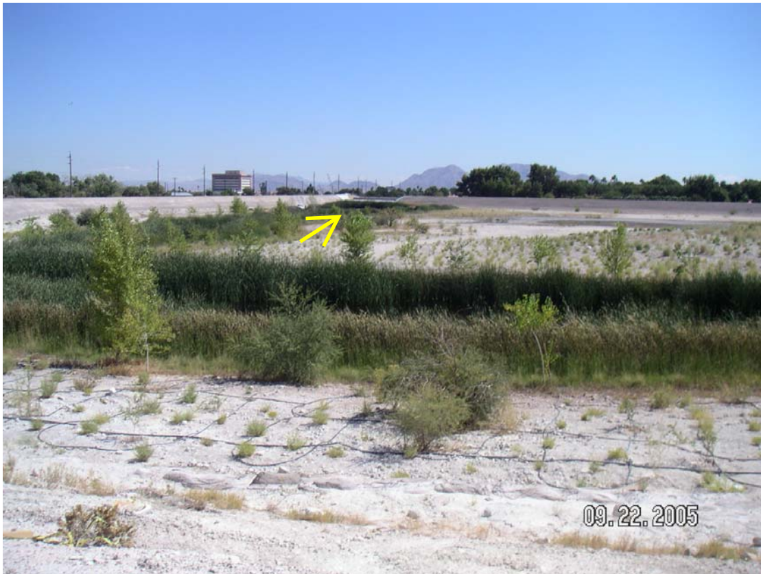
Photo 9. Meadows Detention Basin - outlet area.
