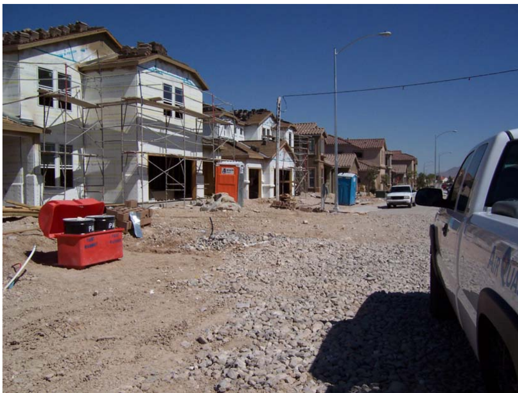
Photo 3. Note portable toilet (blue) in photo right center located immediately adjacent to the paved road upslope of inlets. Note also crush rock for trackout control located in front of pickup truck at photo right.
