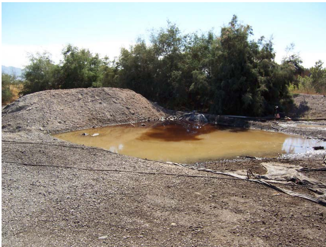
Photo 3. Temporary pit dug to contain wash water from equipment cleaning operation. Note floating oil on the surface of the water.
