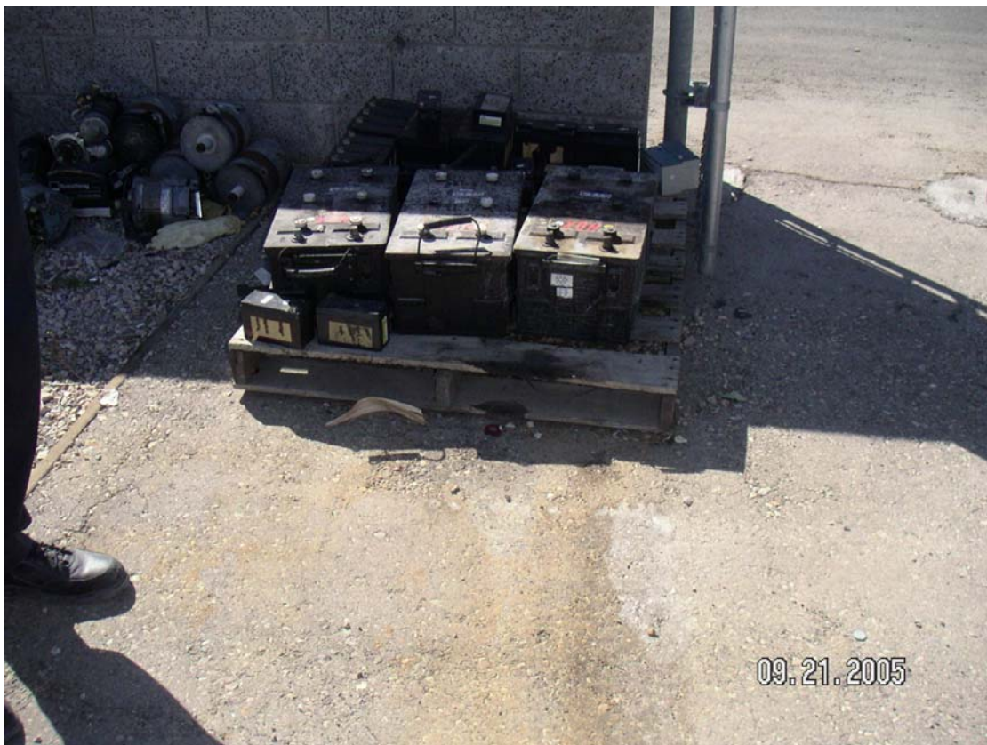
Photo 6. Batteries waiting to be recycled.
