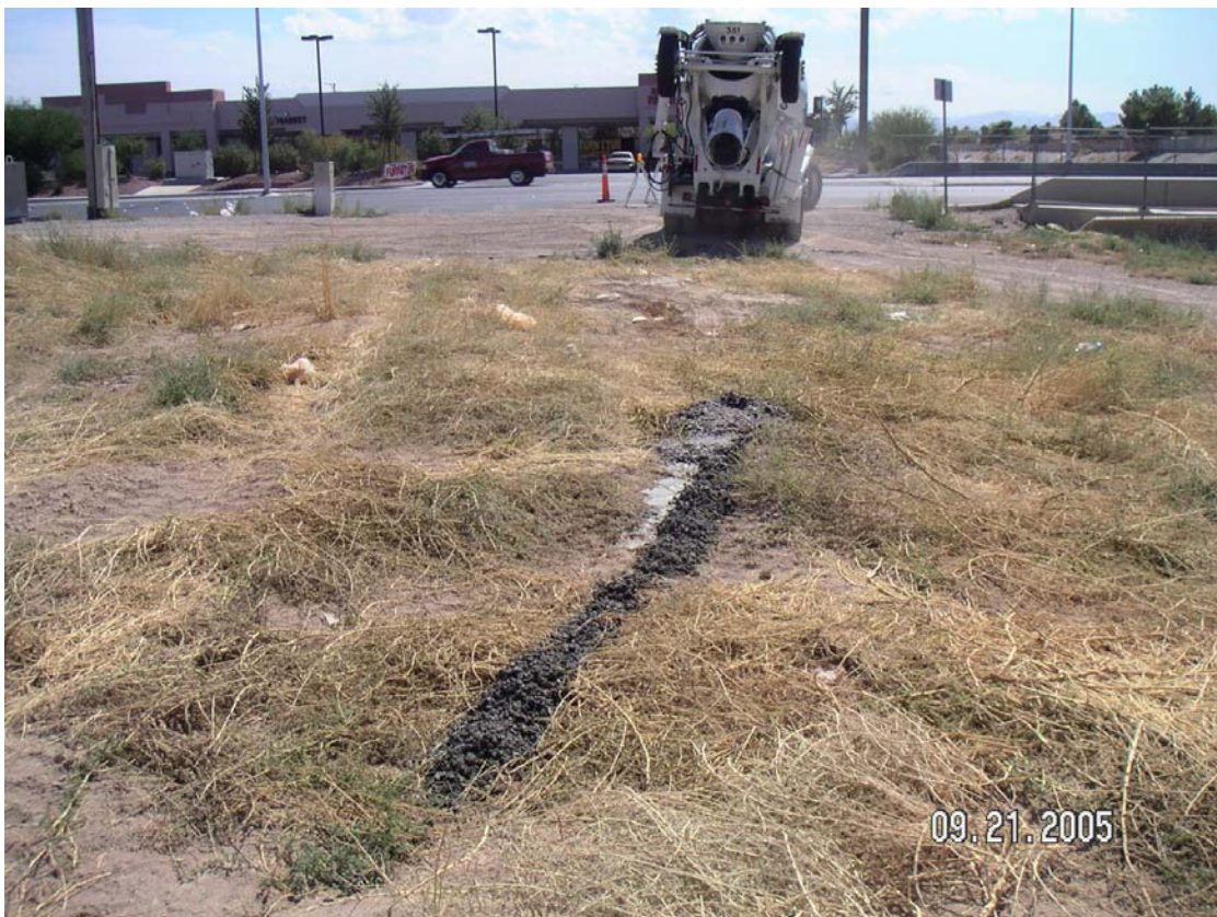
Photo 2. Wash-out material left by concrete truck.
