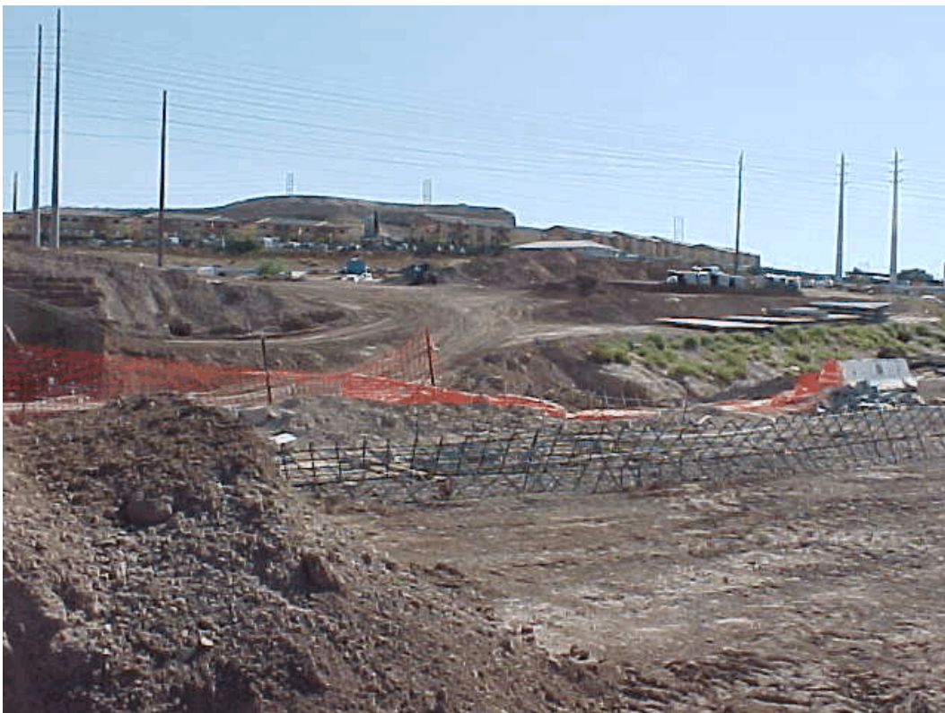
Photo 6. Staging area. Note the soil disturbance and no BMPs.
