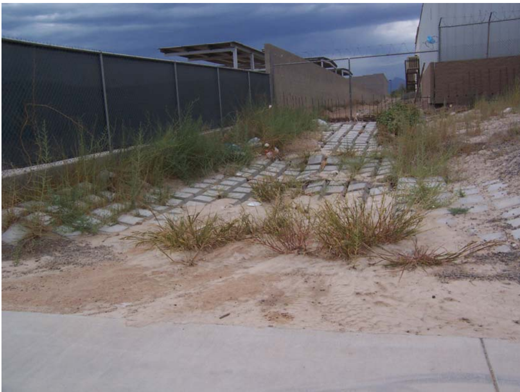
Photo 4. Riprap channel between commercial properties. Note lower end of channel appears to be clogged with sediment.
