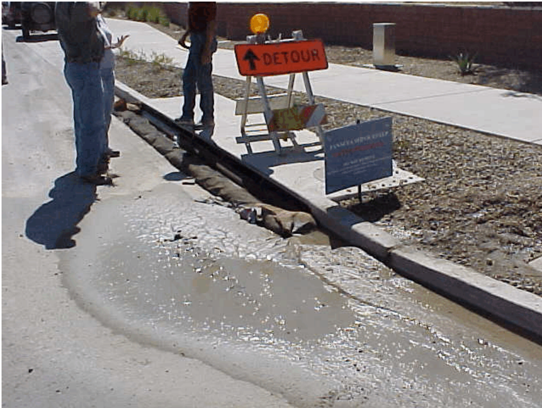
Photo 1. Street inlet protection that is poorly maintained by Landtec LLC.
