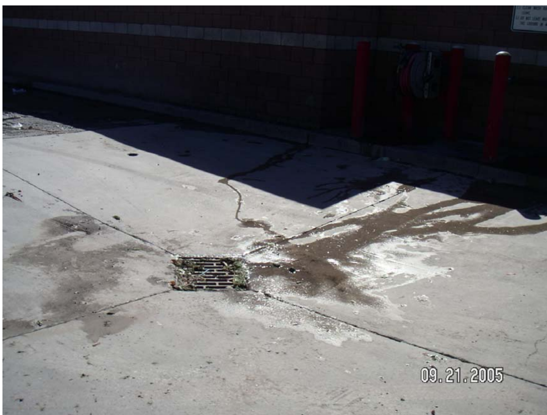
Photo 10. Grate over sand/oil interceptor.
