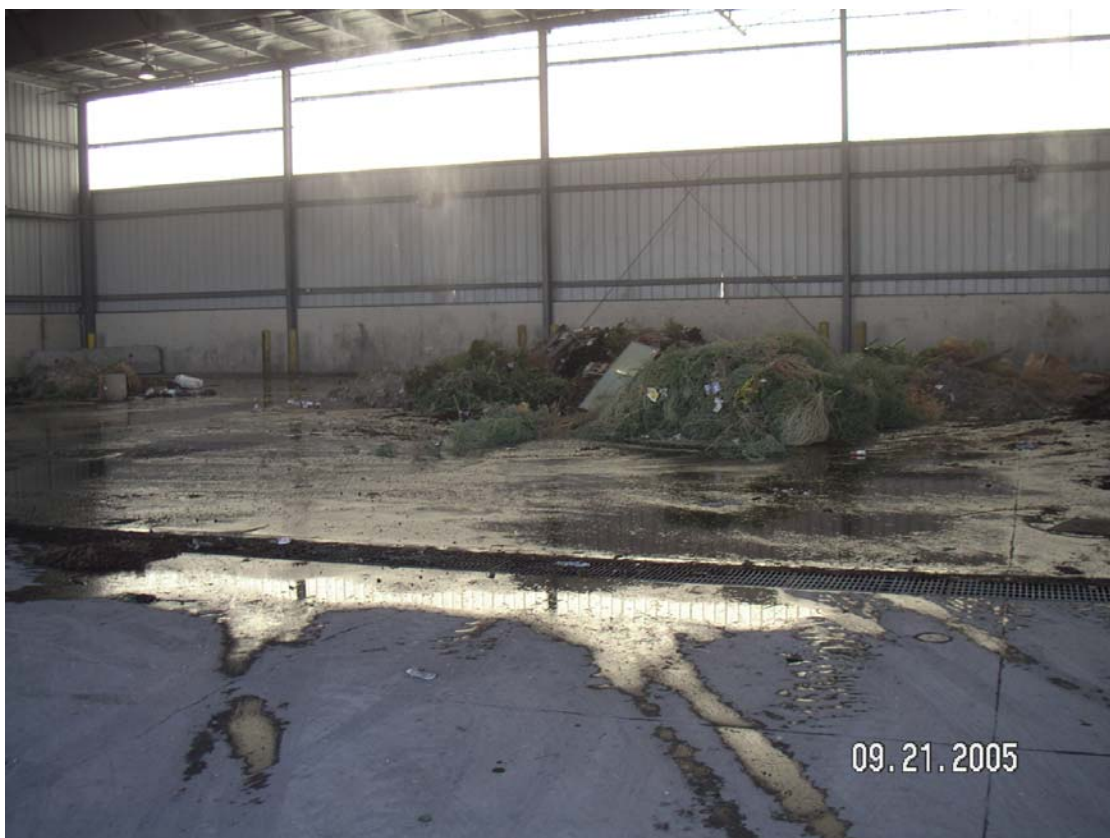
Photo 2. Inside transfer station.
