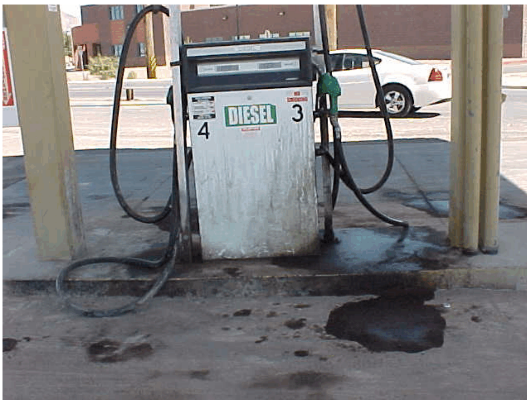
Photo 6. Spillage at fuel island.
