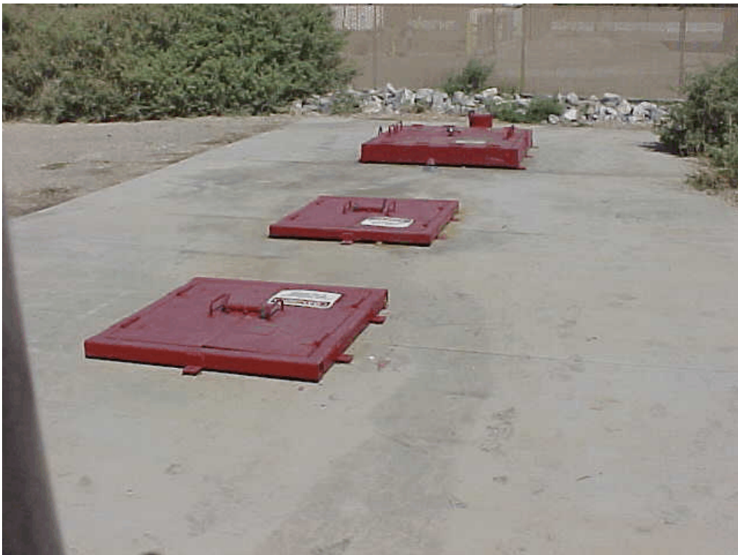
Photo 4. Treatment basin for materials escaping the sediment traps.
