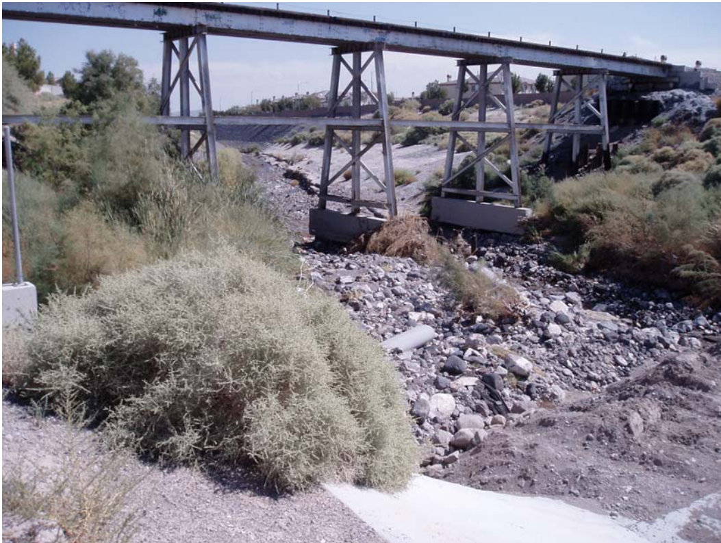
Photo 13. Confluence of Sandwedge Channel, Union Pacific Railroad Channel, and Upper Pittman Wash.
