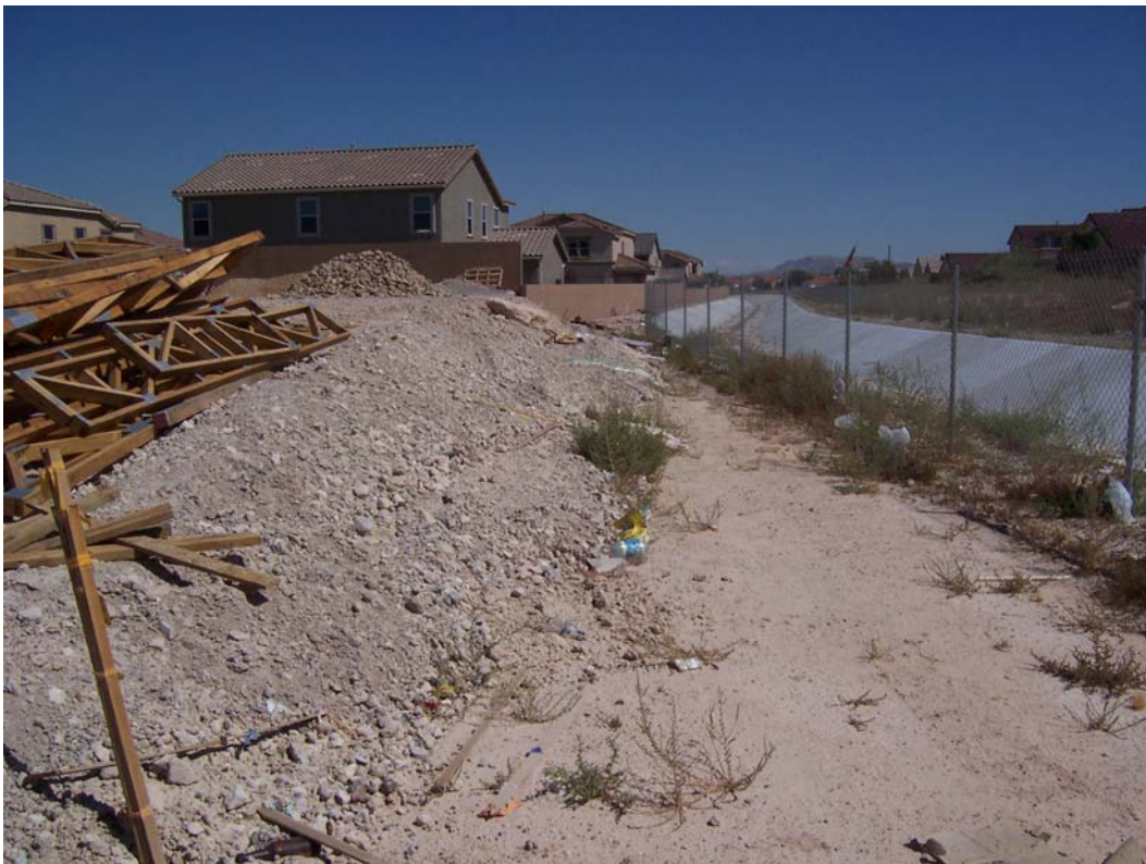
Photo 1. Dirt and debris piled adjacent to wash at the construction site.
