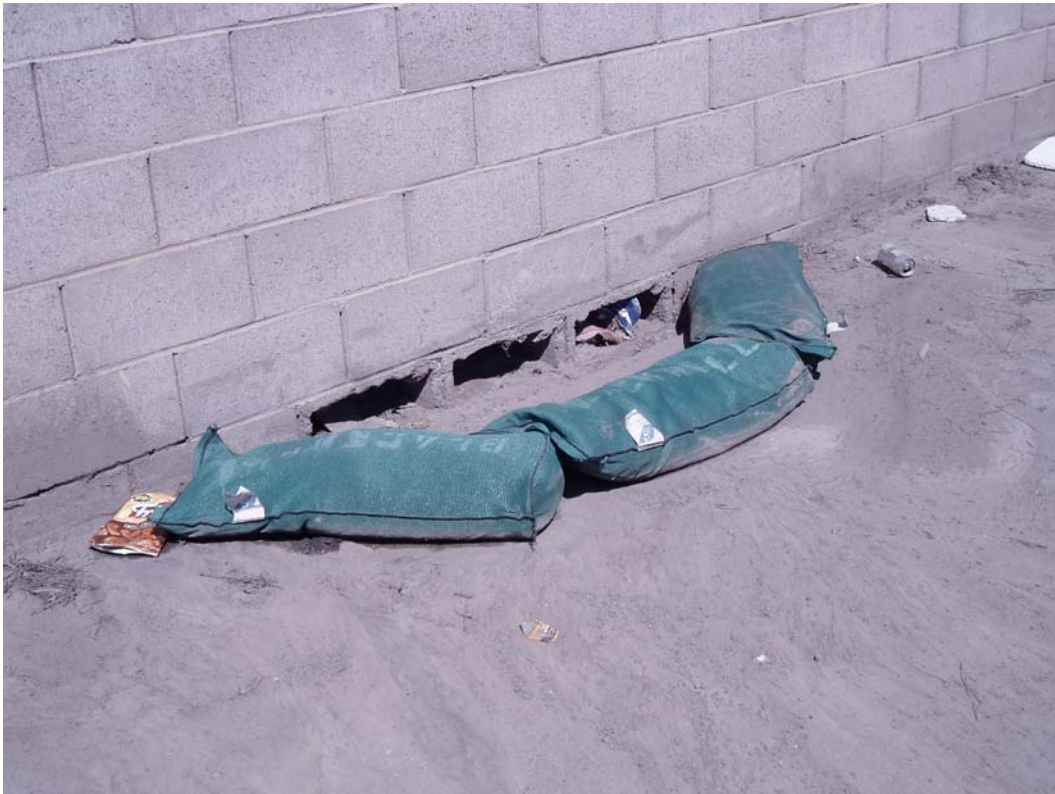
Photo 3. Drain to street in corner of parking lot.
