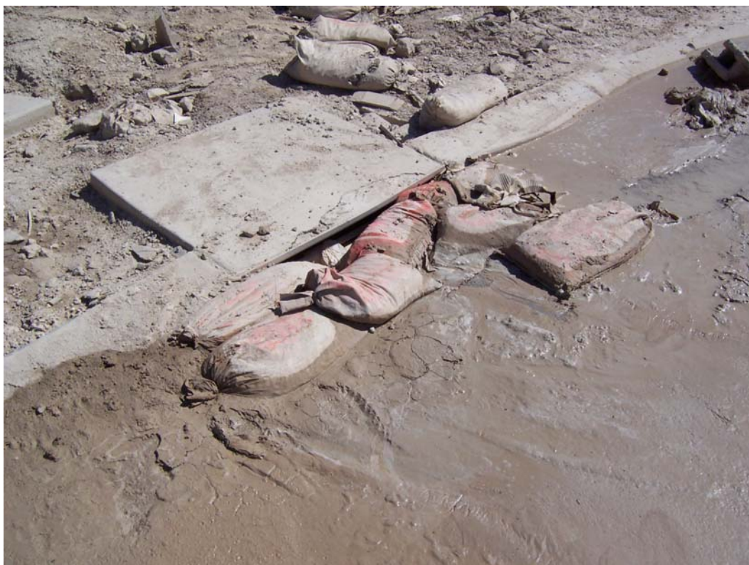
Photo 3. Different storm inlet at the site. Separation between sand bag at the right and curb allows sediment to enter the inlet.
