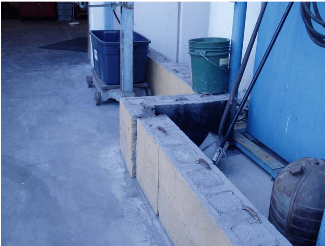
Photo 1. Crack in secondary containment.
