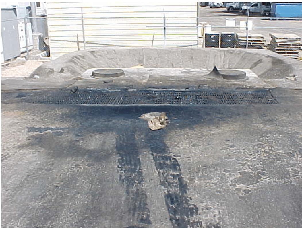
Photo 16. Fleet (secondary) facility: Abandoned asphalt washout area.
