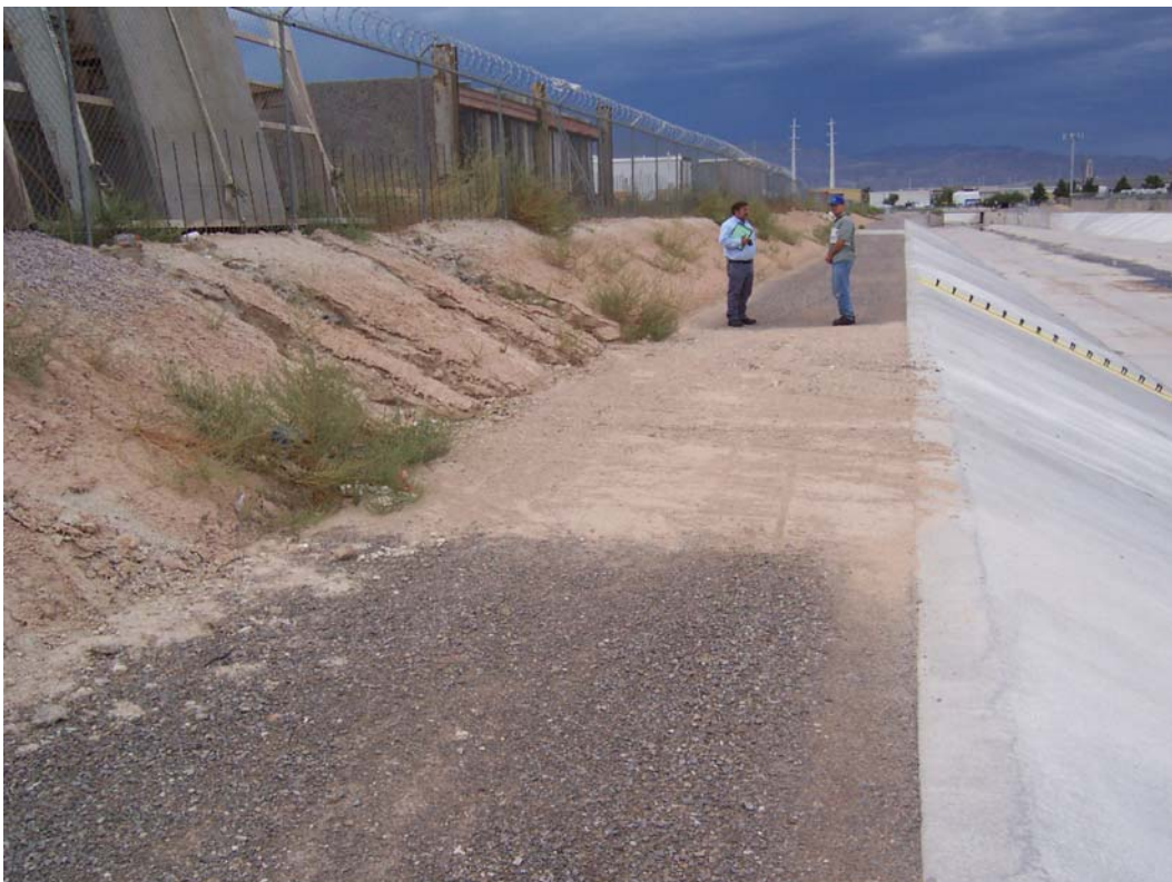
Photo 6. Area where soil erosion on the bank to the left of the wash appears to have entered the wash.
