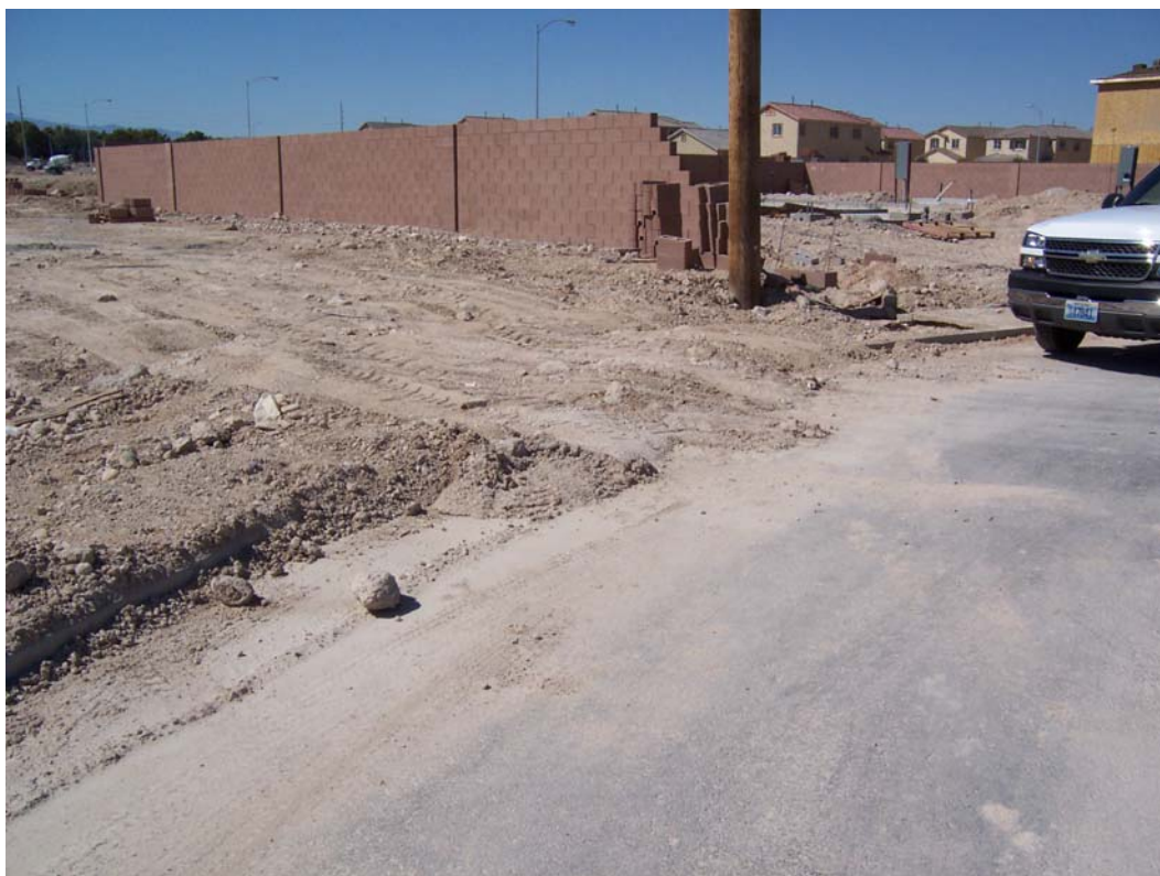
Photo 6. Absence of trackout controls at a site entrance. Note dirt extended past curb line into the street.
