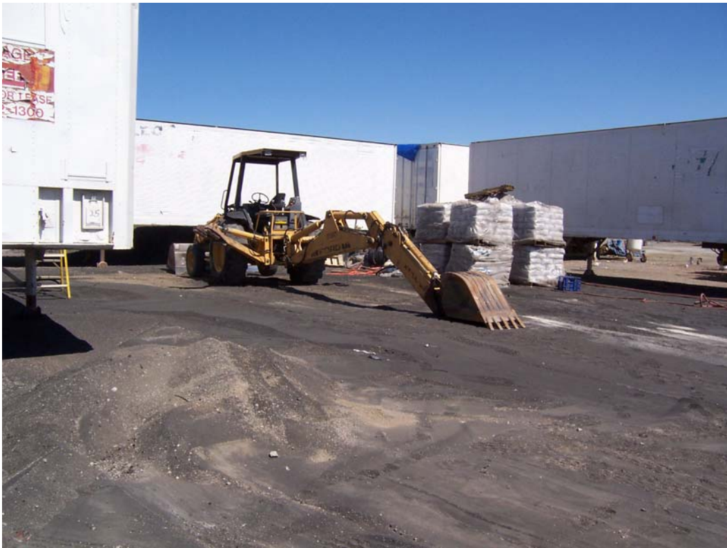
Photo 1. Open air sand blasting activity at the site. Dark material around the backhoe being sand blasted is spent sand blast grit. White bags on pallets at photo right are additional unused grit. No containment was provided around the area.
