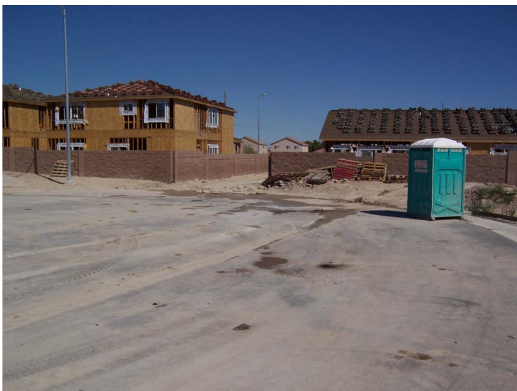
Photo 4. Portable toilet placed where spillage would go directly to storm inlet. Storm inlet is left center photo, at the end of the sidewalk to the cul-de-sac.
