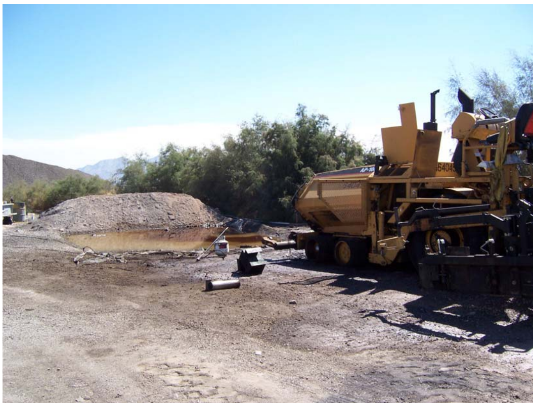
Photo 4. Paving machine being cleaned with wash water discharged to the pit shown in Photo 3. Note oil stains on the ground in front of and around the machine.
