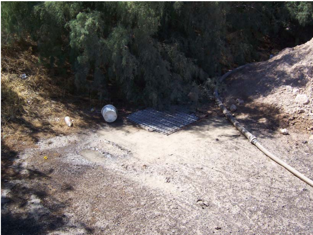
Photo 5. Storm inlet located behind the pile of dirt shown in Photos 3 and 4. Note contaminated runoff from the site entering the inlet.
