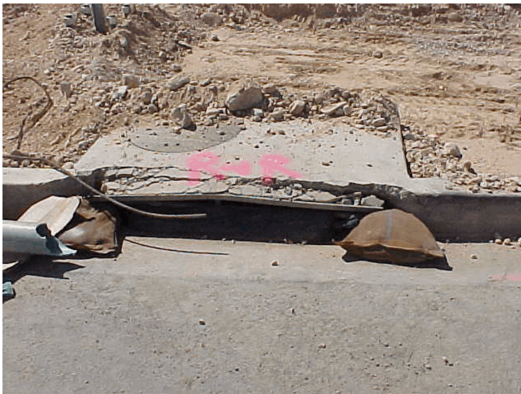
Photo 3. Street inlet protection that is poorly maintained by Landtec LLC.
