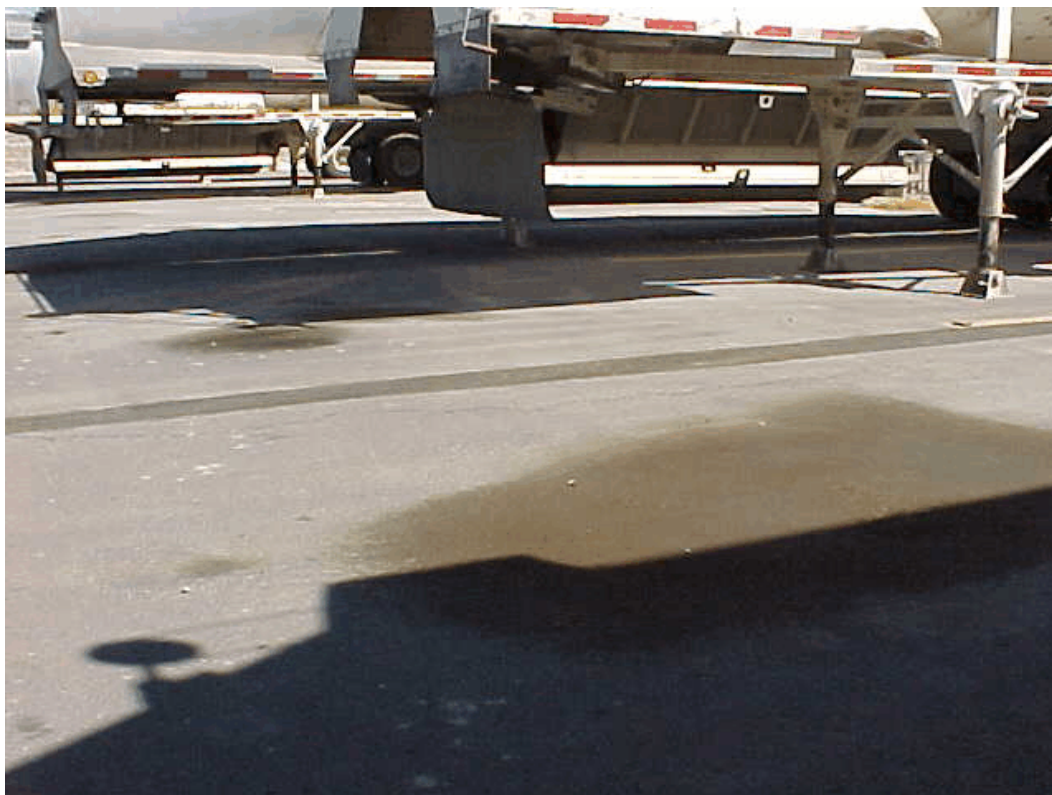
Photo 13. Fleet (secondary) facility: Truck and paving equipment parking area with spills/leakage staining on pavement.
