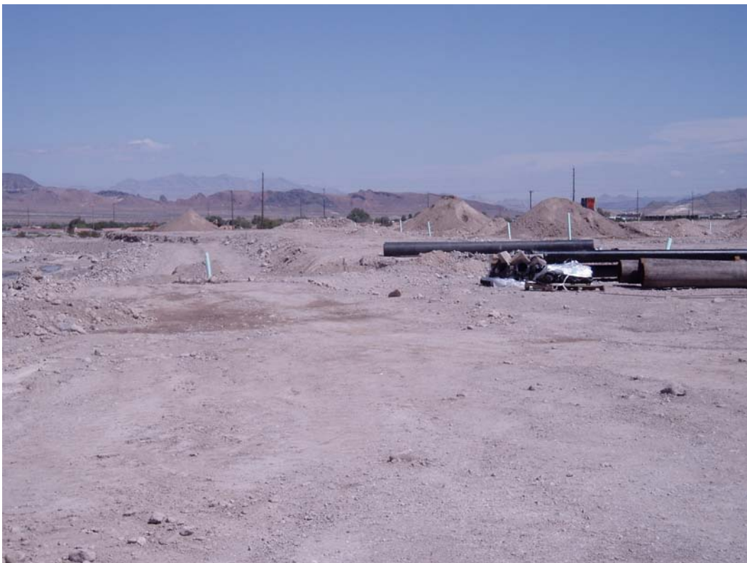
Photo 26. Construction and sediment piles (photo right) adjacent to Gibson Channel (photo left).
